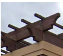
8 WOOD PERGOLA BROWN TEAK WOOD REF. MATCH EXISTING SHIPPING CENTER REF. COLOR CUSTOM BROWN SEE 3/A-400
