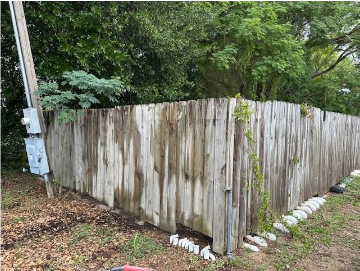
Outside Equipment Compound, North Side, and partial West Side with remedial well points on Standby for Small System, Facing SE
