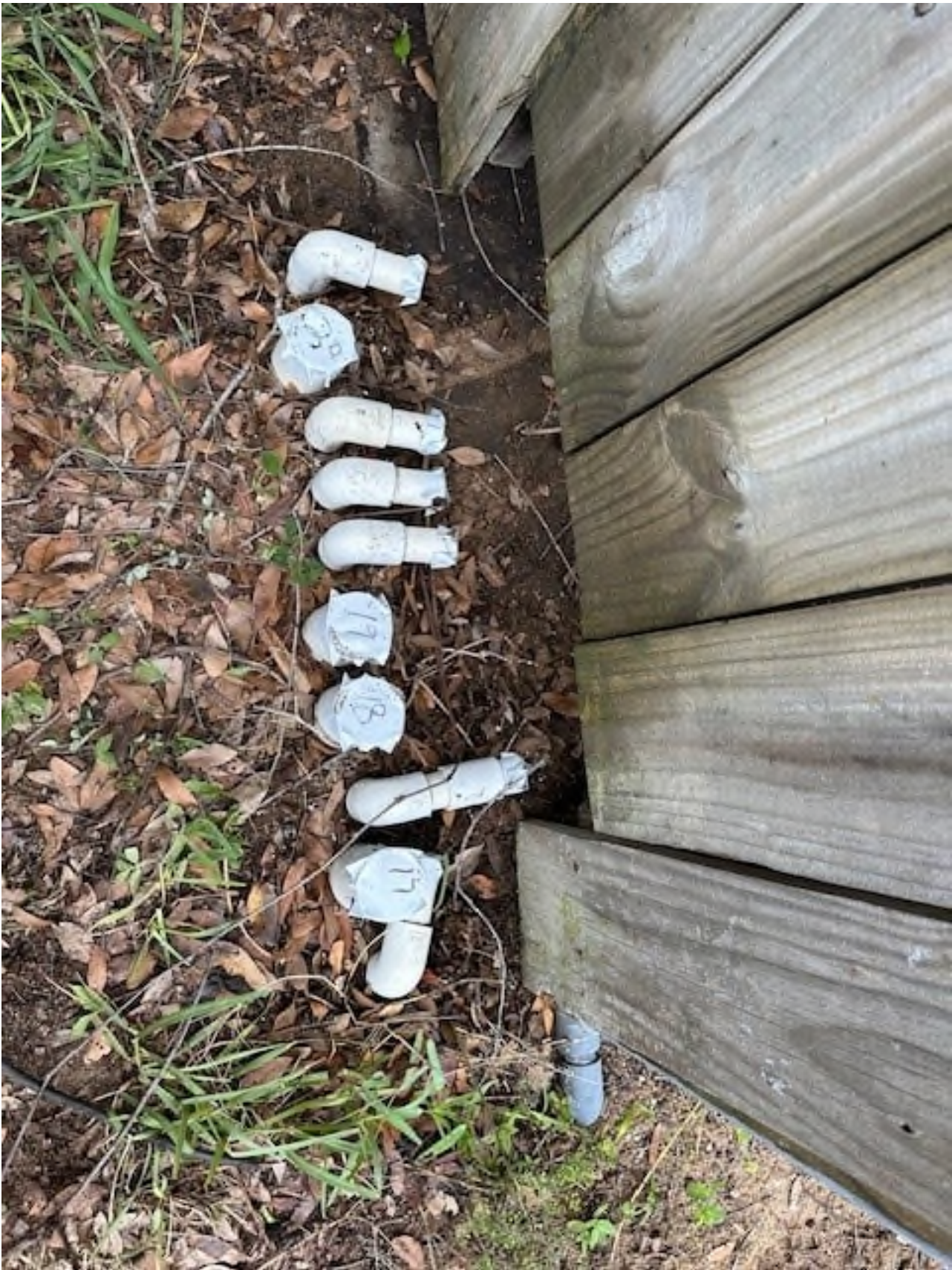
Covered Remedial Wells Points for AS-25 to 30 and EW-17 to 20, along North Side of Equipment Compound, placed in West to East Direction from Compound NW Corner.
