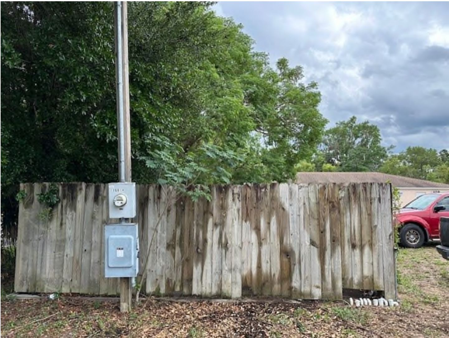
Outside North Side Equipment Compound, with 3-phase, 240V, 200A Service Pole, facing South
