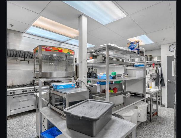
COMMERCIAL KITCHEN Full build-out, hooded cook line
