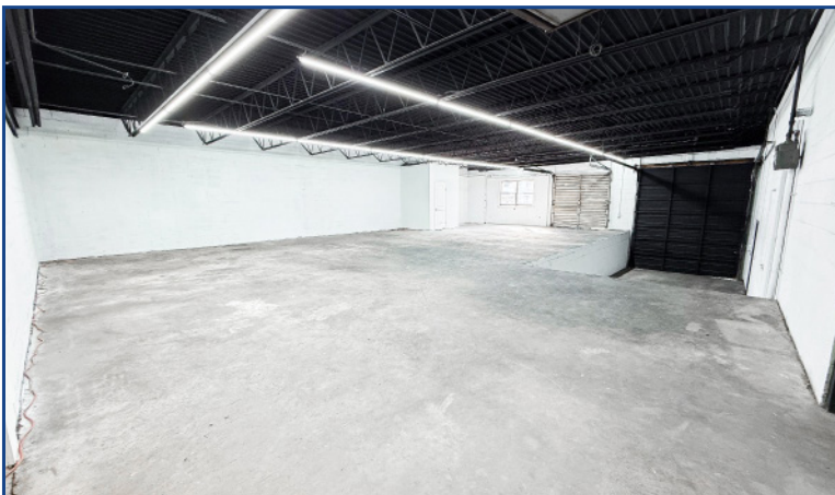
LED LIGHTING THROUGHOUT
