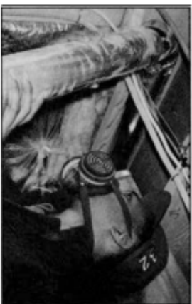
Heating and air conditioning ducts can accumulate dust that contains lead.
