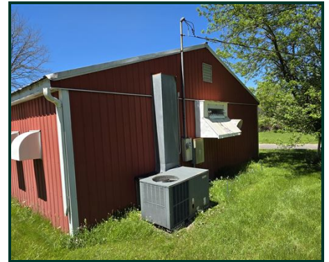
Building exterior — awning ventilation
