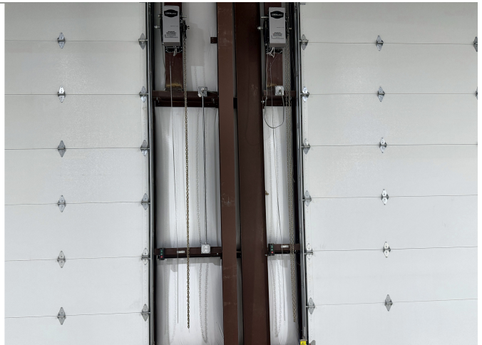
Overhead doors — 14' x 14' grade-level with powered openers
