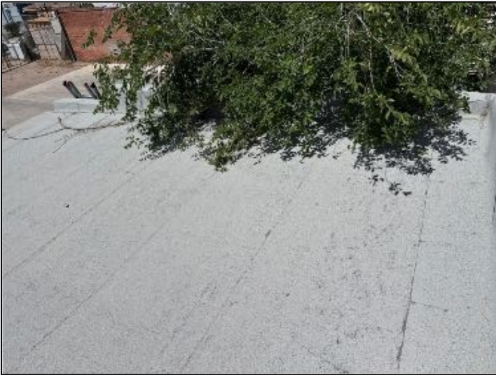
Tree branches were touching parts of the detached structure roof, which has caused damage to roof top material. Recommend trimming back of ALL tree branches and correction to roof top material
