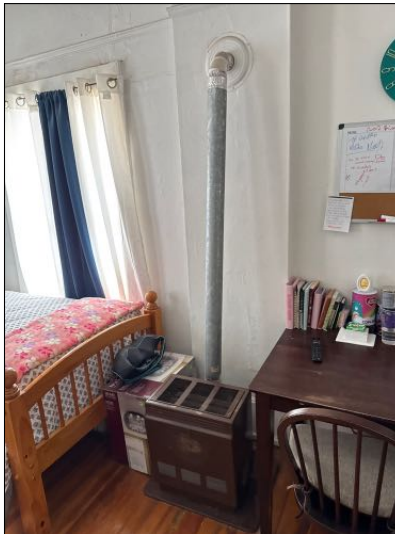
Unit 2 bedroom showed to have a space heater
