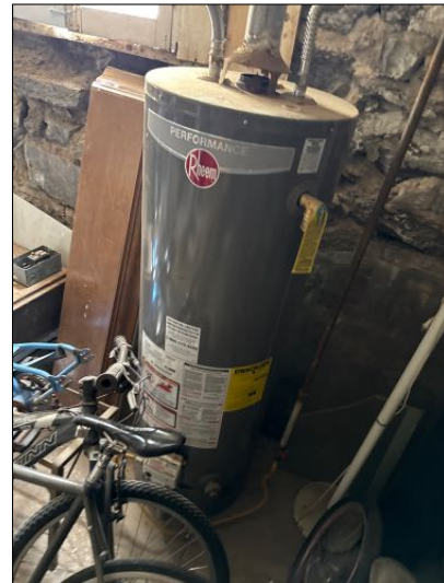
Water heater was functional as need be
