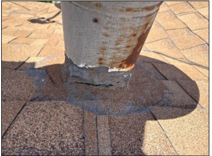
Another representative example of unsealed roof top protrusions
