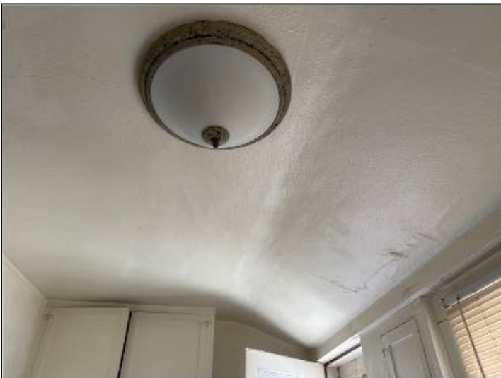
View of cracks in unit one kitchen ceiling
