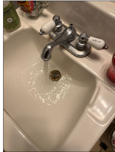
MAINTENANCE:unit 3 bathroom sink plumbing drained slow, recommend repair and or correction
