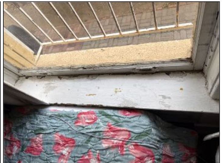
SAFETY CONCERN: Various windows were painted shut. Recommend correction as to allow proper function and safety for proper egress
