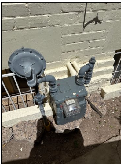
View of gas meter
