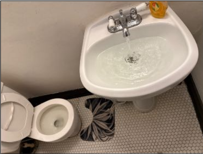
MAINTENANCE:unit 1 bathroom sink plumbing drained slow, recommend repair and or correction
