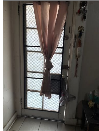
Sunlight showed to be entering through cracks of unit 4 door
