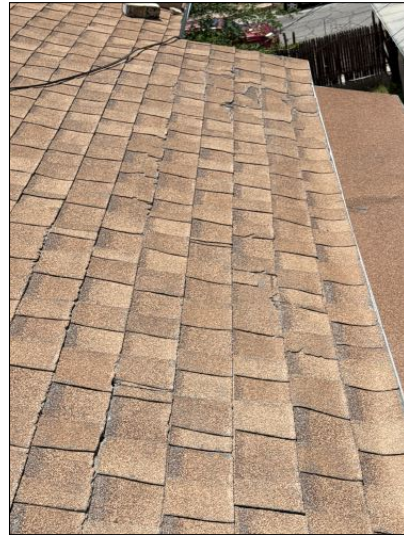
Damaged roof material, various shingles showed wear, loss of granules and or damaged shingles on backside of roof. Recommend correction
