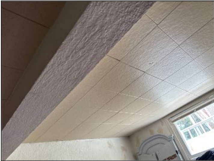
SAFETY CONCERN: Ceiling tiles in unit 5 may be Asbestos-Containing Material (ACM,) and if "handled" or otherwise "disturbed," a qualified environmental specialist should be consulted."
