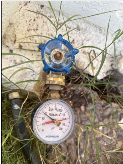
Static Water Pressure Reading: 60psi
