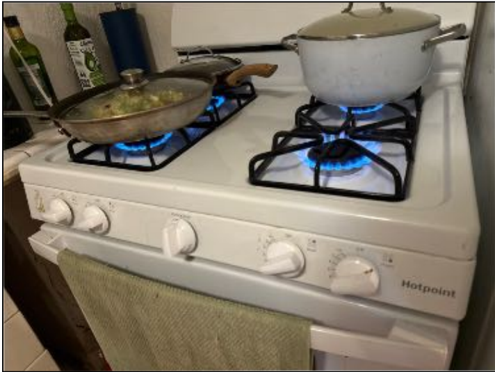
Unit operated normally (cook top): unit 5
