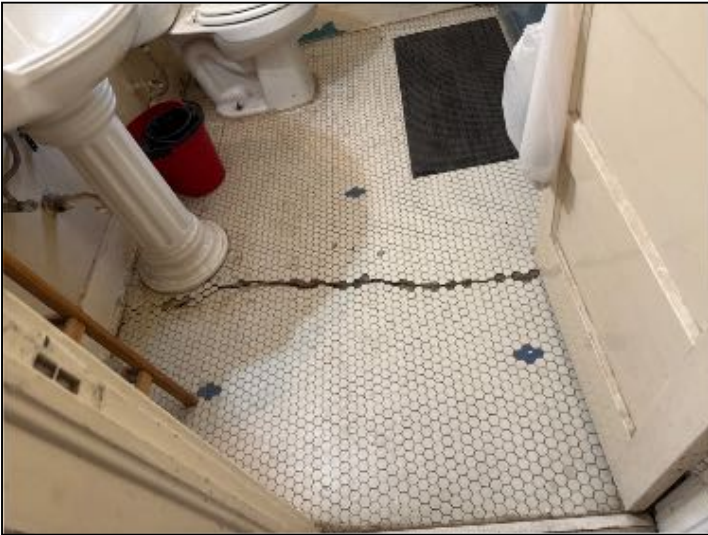
View of cracks in unit 4 bathroom floor
