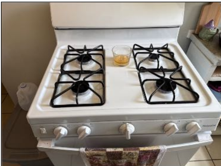
Unit operated normally (cook top): unit 3
