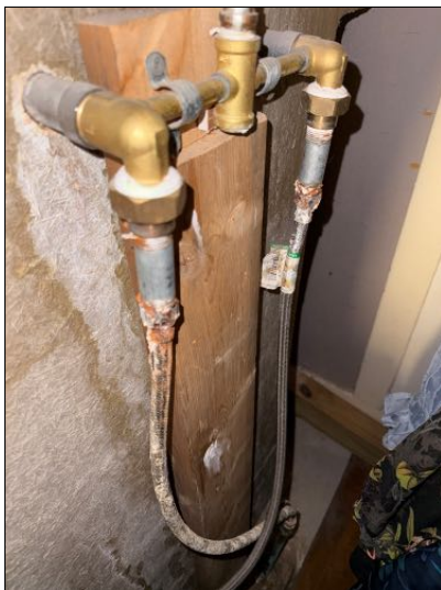
MAINTENANCE:Corrosion of water pipes in unit 3 bathroomseemed to be evident, recommend repair and or correction
