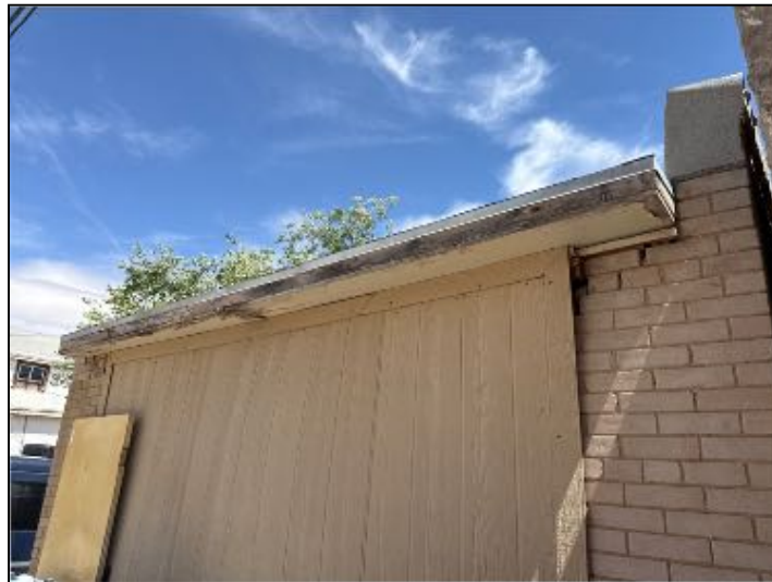
View of weathered, fascia, and soffits on detached structure
