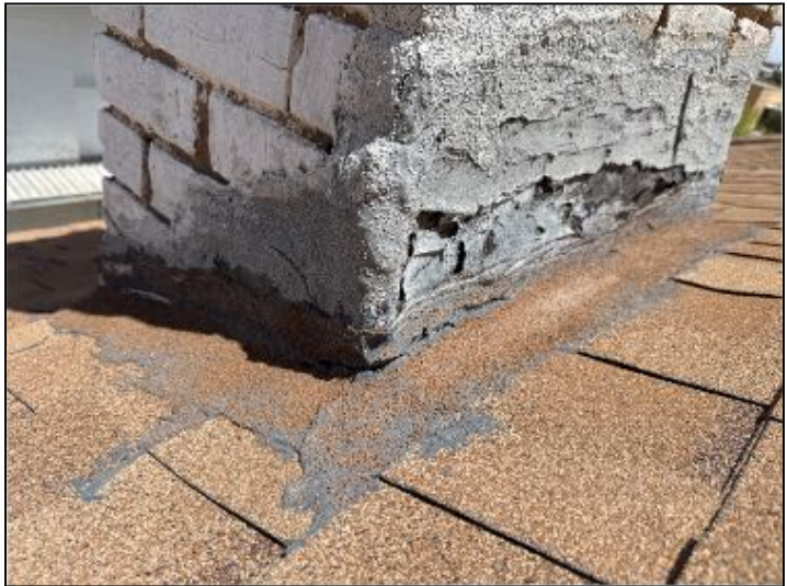
MAINTENANCE: Recommend resealing ALL cracks and crevice on roof top material.
