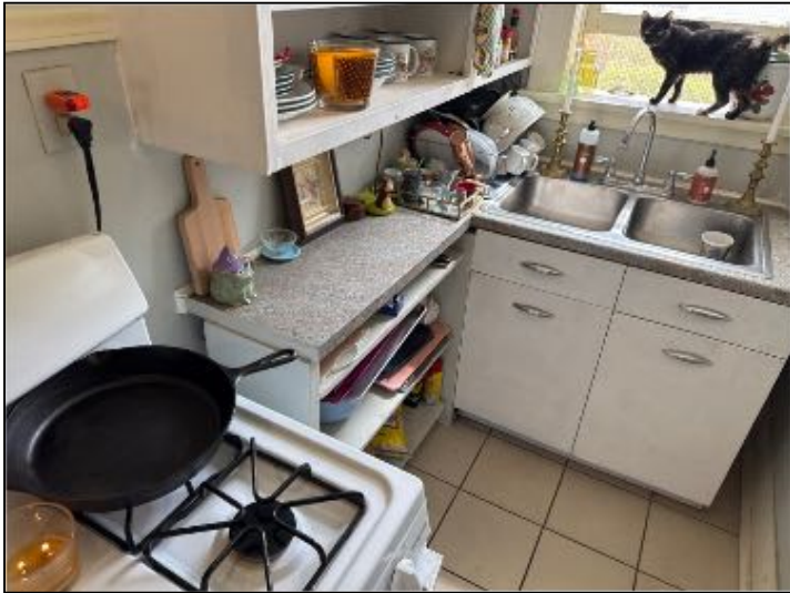
Outlets within 6 feet of kitchen sink, not GFCI
