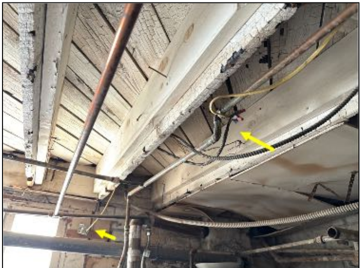
Another representative example of missing junction box cover in basement
