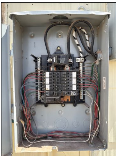
Main electrical panel with shut off
