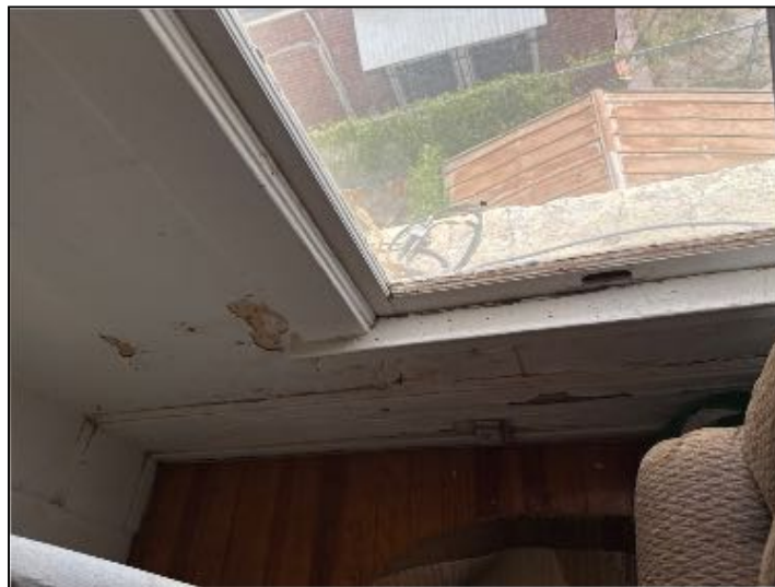
View of previous water damage to walls in unit 2
