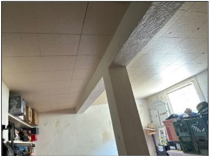
SAFETY CONCERN: Smoke detectors were missing in Bedrooms . Recommend correction as to allow proper function: all units
