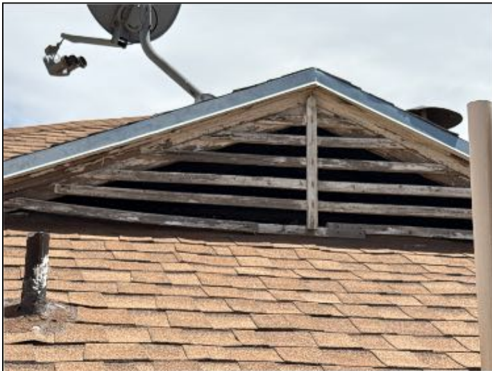
MAINTENANCE: Weathered wood was evident on various areas of structure. Recommend correction.
