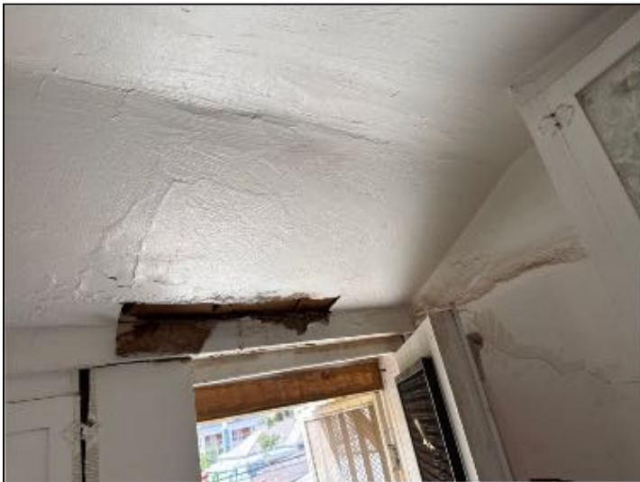
View of previous water intrusion and damage to ceilings in Unit 2 area of structure
