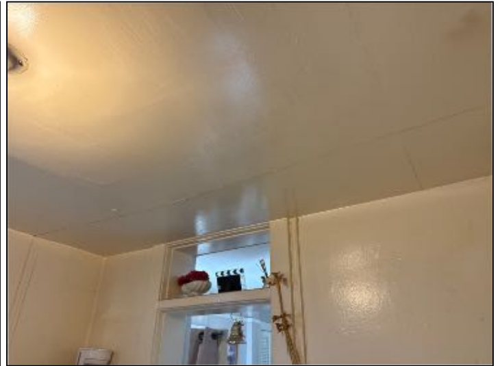
View of cracks in unit 4 kitchen ceiling
