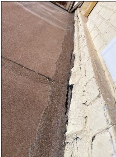
Another representative example of cracks and crevice on roof top material
