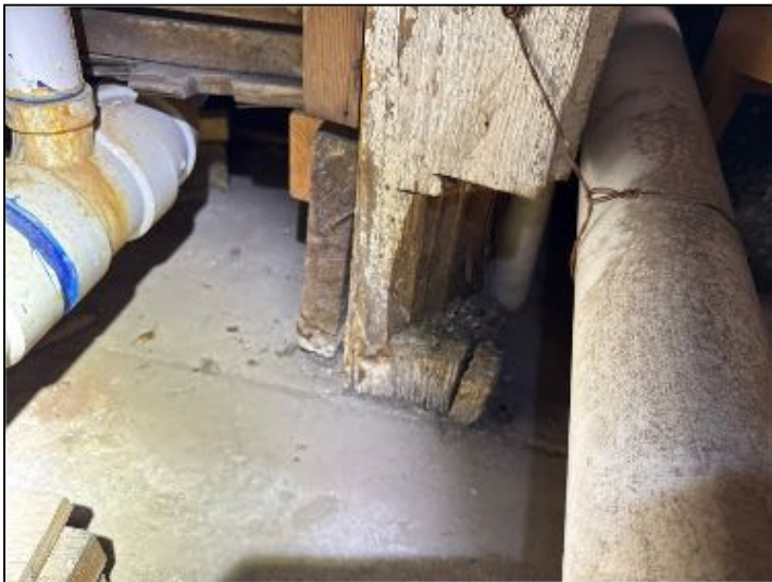
IMPROVE: A 4x4 wood column in basement showed to be overly notched. Recommend further evaluation and correction.
