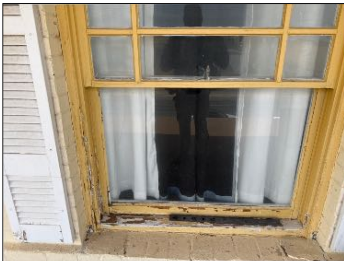
SAFETY CONCERN: front window showed to be broken. Recommend replacement of ALL defective windows
