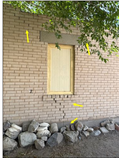
View of detached structure with crack in foundation stem wall going up alongside brick. Recommend further evaluation and correct correction.
