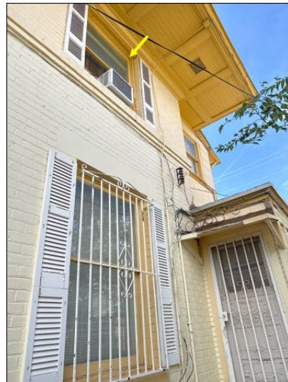
SAFETY CONCERN: rightside upstairs window showed to be broken. Recommend replacement of ALL defective windows
