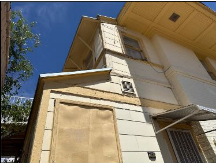
Another representative example of weathered wood on left side of structure walls
