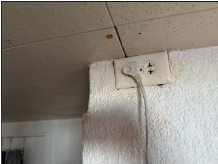
IMPROVE:"TWO-prong outlets" receptacles (no equipment ground) throughout structure. This is a common problem in a home of this age when 2-wire Romex is present without an equipment ground. Recommend further evaluation for different types of corrections and allow proper safety and function
