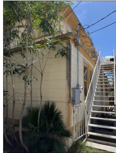
Another representative example of weathered wood on back of structure walls
