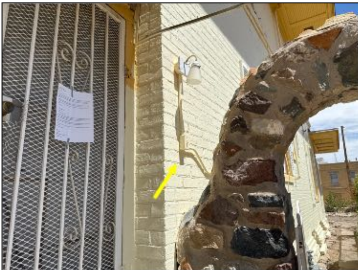
MAINTENANCE: Exterior switch was missing weather poof cover. Recommend correction
