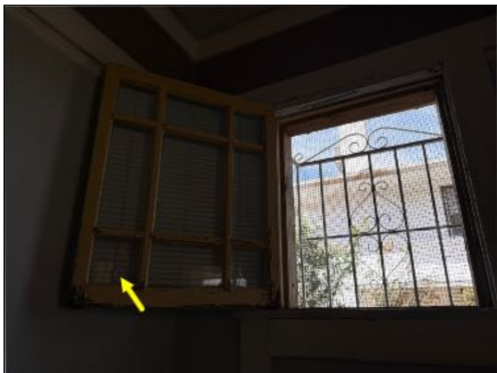
SAFETY CONCERN: unit 3 window showed to be broken. Recommend replacement of ALL defective windows
