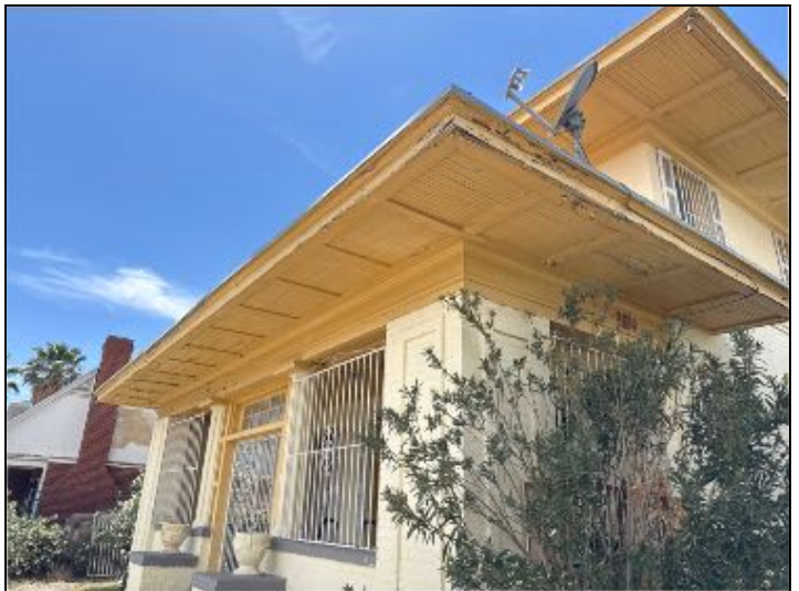
Another representative example of weathered, soffit, fascia, and eaves on front of structure
