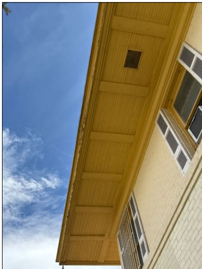
MAINTENANCE: Various areas of soffits, eaves and Facias showed evidence of water damage, recommend correction.
