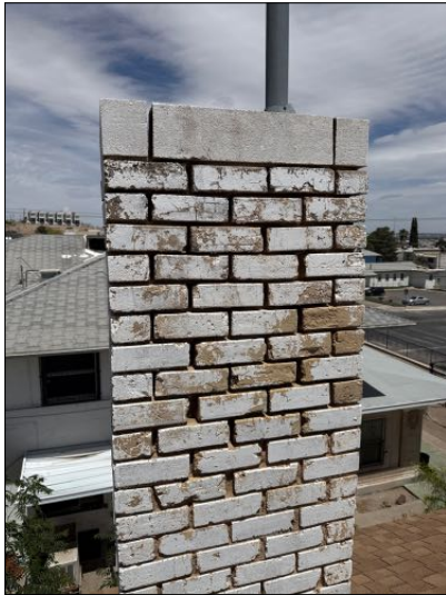
View of cracks and crevice on chimney structure walls
