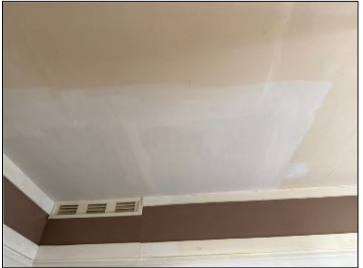
View of previous repairs to ceilings in Unit 3 area of structure
