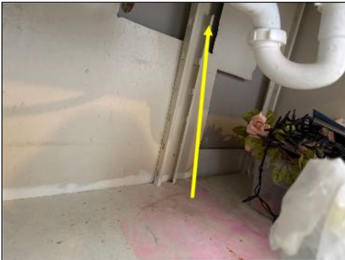
MAINTENANCE: Plumbing for unit 3 kitchen sink showed to be actively leaking, recommend correction as to prevent excess moisture.
