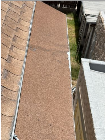
MAINTENANCE:Roof material showed to have been improperly placed from drip edge. Recommend correction.
