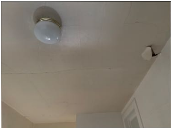
View of previous water intrusion and damage to ceilings in foyer hallway area of structure
