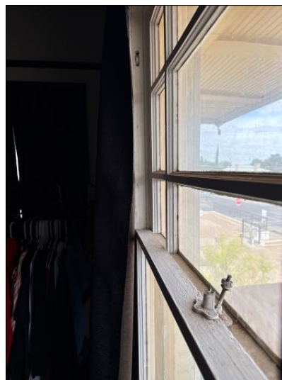
MAINTENANCE: Various windows showed to have defective hardware. Recommend correction to ALL defective windows
