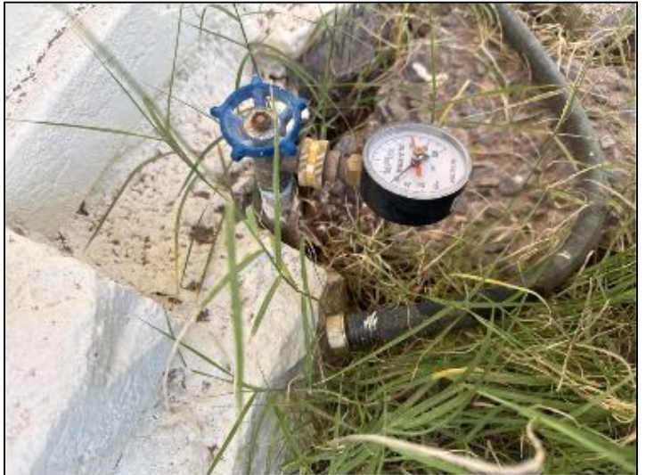
MAINTENANCE:Recommend back flow prevention nozzle on all exterior hose bibs
