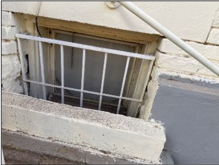
SAFETY CONCERN: rightside bottom window showed to be broken. Recommend replacement of ALL defective windows
