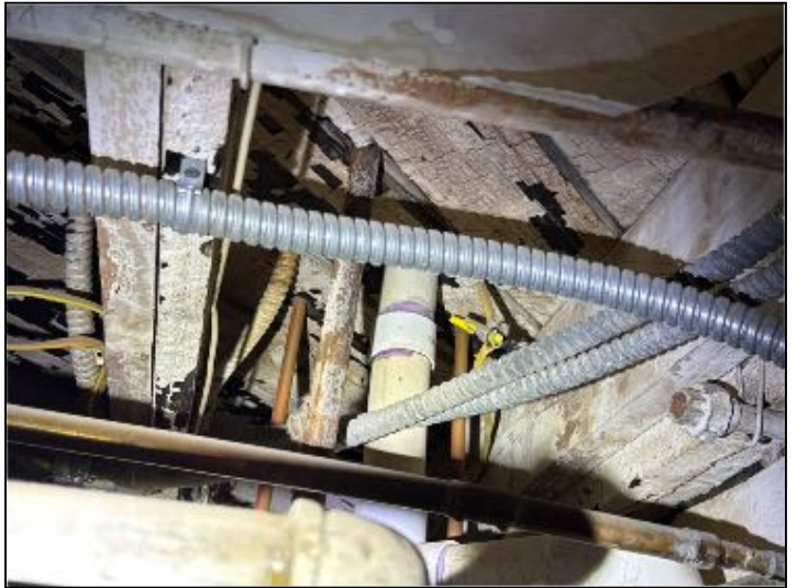
IMPROVE: Junction box was missing cover in basement . Recommend correction as to allow proper safety and function
