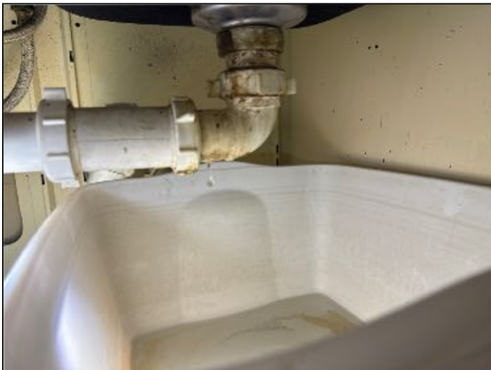
MAINTENANCE:Plumbing for unit 5 kitchen sink was leaking, recommend correction as to prevent damage, excessive moisture.
