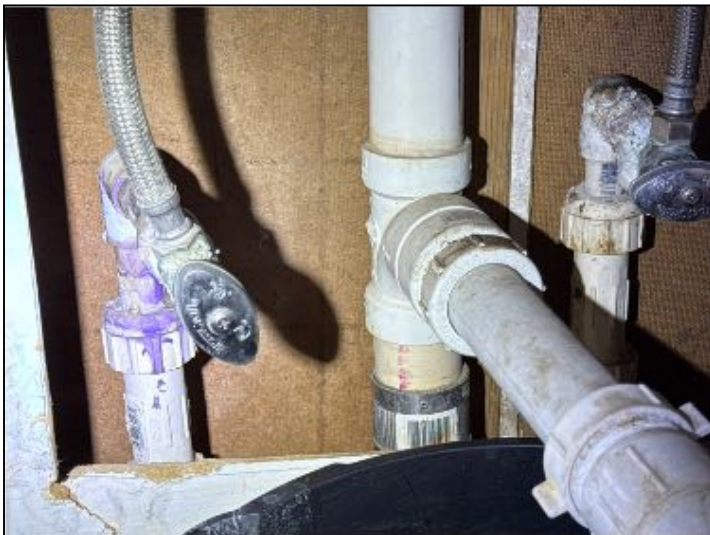
IMPROVE: unit 2 hot water supply showed to be using PVC. Recommend proper hot water type material.
