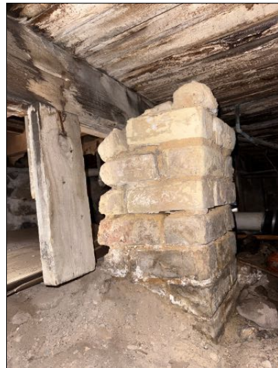
Addition foundation structure showed to be lacking support. Sloped floors, cracks in floors, walls and ceilings in unit 4 were evident. Recommend a structural engineer for further details and correction
