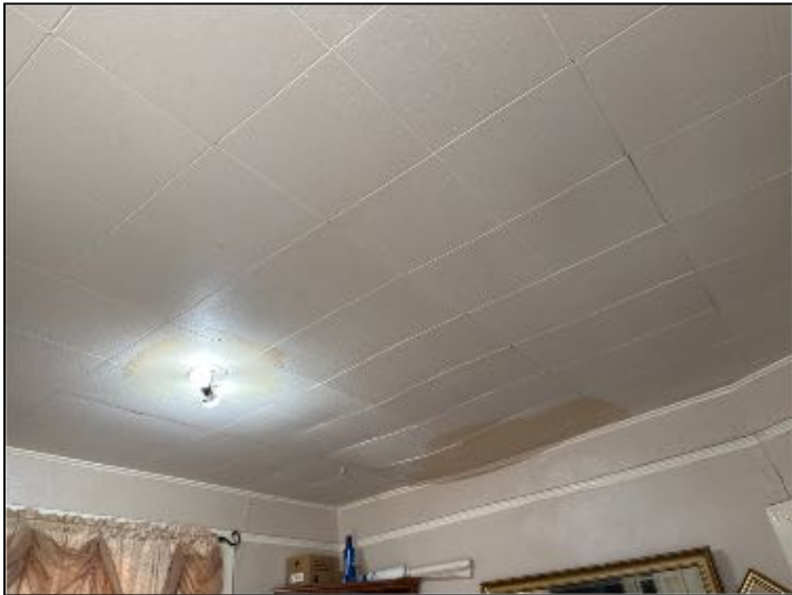
View of previous repairs to ceilings in Unit 4 area of structure
