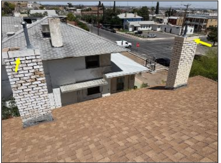
View of cracks and crevice on chimney structure walls
