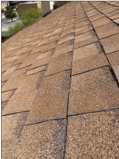
Another representative example of hail damage on roof top material
