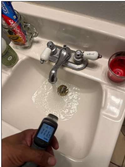
Water heater was functional as need be
