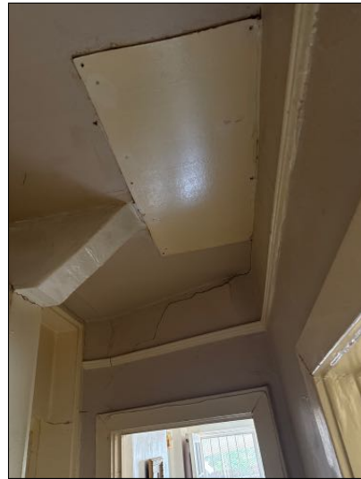
View of cracks in unit 4 hallway, ceiling and walls
