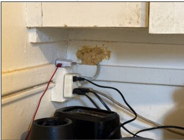
SAFETY CONCERN:Extension cord showed to be going through wall from unit 4 kitchen. Recommend correction with proper type wiring and conduit as to allow proper safety and function
