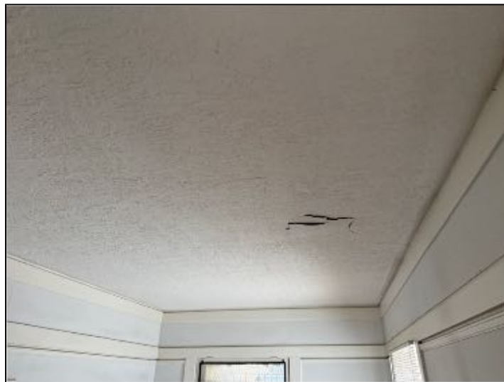
View of cracks in foyer ceiling drywall
