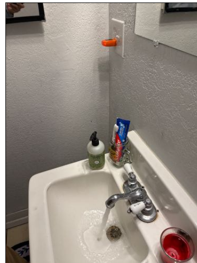
Bathroom outlets, not GFCI
