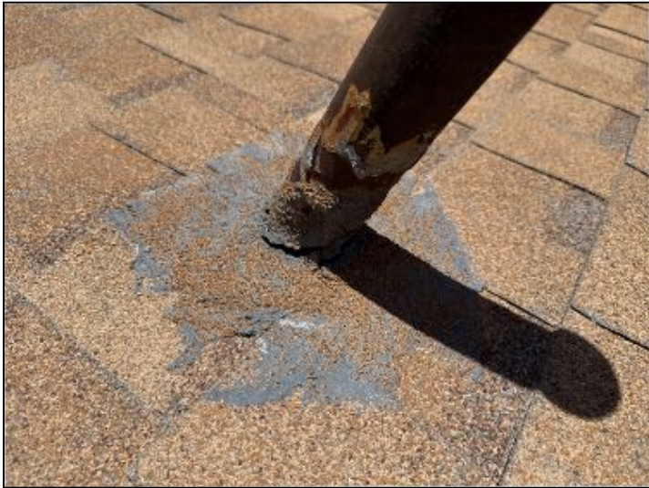
MAINTENANCE: Recommend re-sealing of ALL protrusions through the roof.
