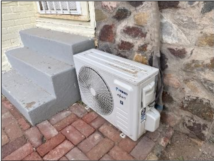
View of AC unit
