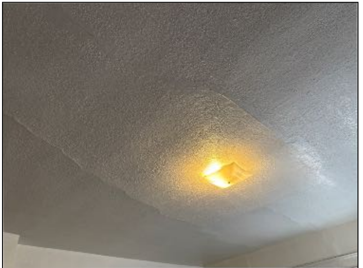
View of cracks in unit two bedroom ceiling
