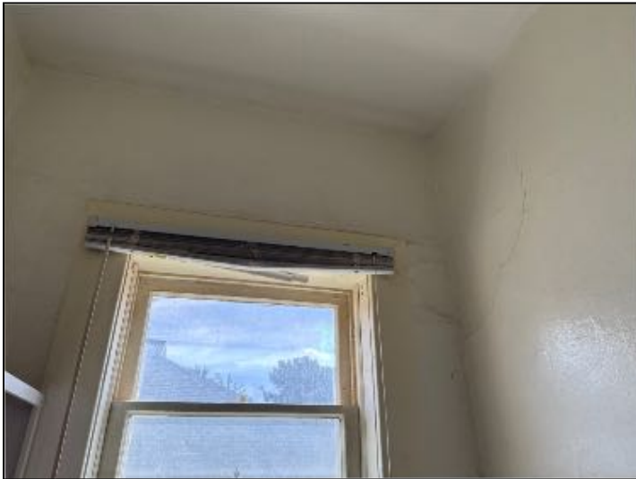
View of cracks in walls over unit 3 kitchen window
