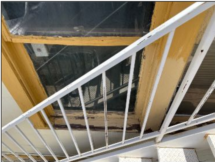
MAINTENANCE: Weathered wood was evident around various window frames. Recommend correction as to prevent further damage.
