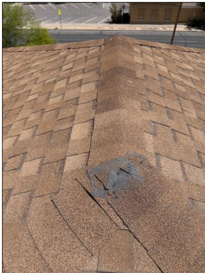
MAINTENANCE: Exposed nails were present on roof top material. Recommend sealing of ALL exposed nails on roof top
