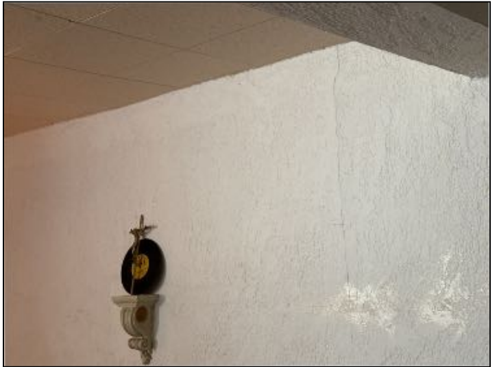
View of crack in unit 5 wall bedroom
