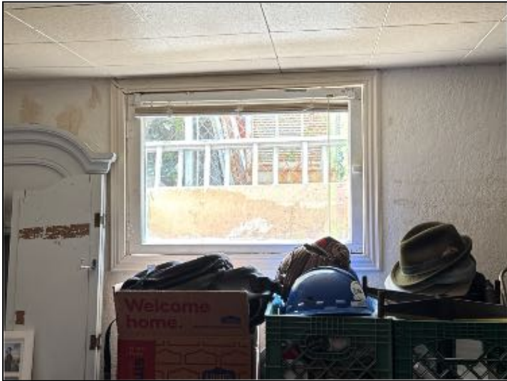
MAINTENANCE: Recommend sealing around interior window frame walls. As to allow proper efficiency
