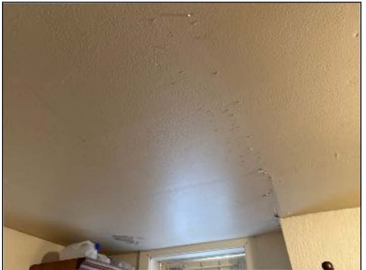
View of previous water intrusion and damage to ceilings in Unit 5 area of structure
