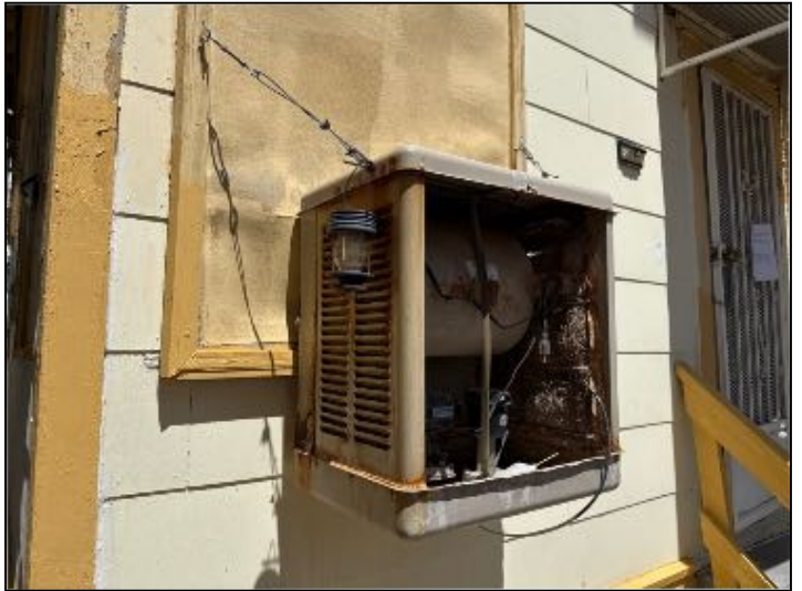
Back leftside unit: inoperable
