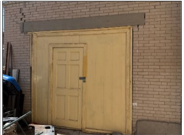
Another representative example of weathered wood on detached structure walls
