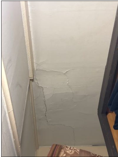
View of previous water intrusion and damage to ceilings in Unit 3 Closet area of structure
