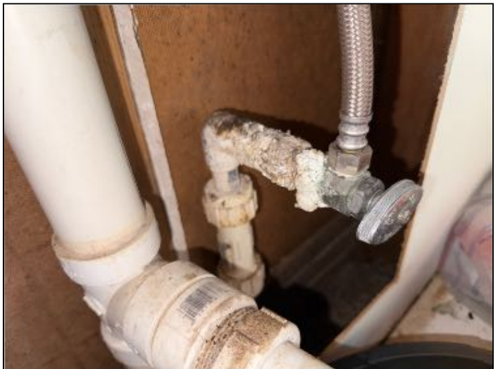
MAINTENANCE: Corrosion of water pipes in unit 2 kitchen seemed to be evident, recommend repair and or correction
