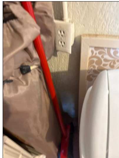
IMPROVE:Tamper resistant type receptacles less than five & one half feet above floor were not present throughout structure. Recommend placement.
