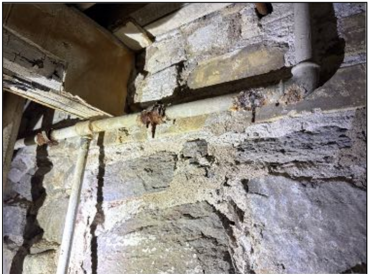
MAINTENANCE: Plumbing for basement galvanized water line showed to be actively leaking, recommend correction as to prevent excess moisture.
