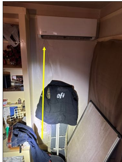
IMPROVE: unit 4 mini split showed to be leaking condensation into bedroom. Recommend correction.
