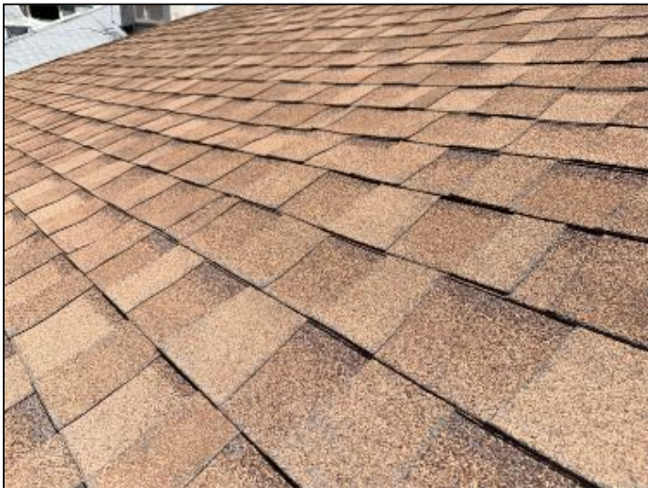
Hail damage was evident on roof top material. May allow further rapid deterioration of material, water intrusion and or moisture related issues. Recommend further evaluation by roofer
