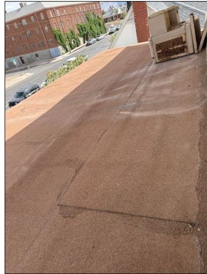
Ponding on rolled roofing areas were evident. Recommend further evaluation and correction.
