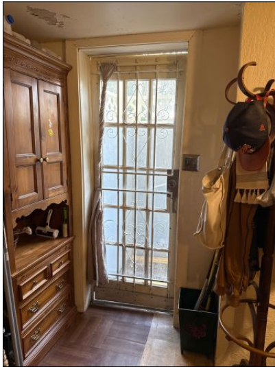
Sunlight showed to be entering through cracks of unit 5 door
