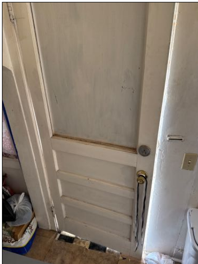
Sunlight showed to be entering through cracks of unit 1 door
