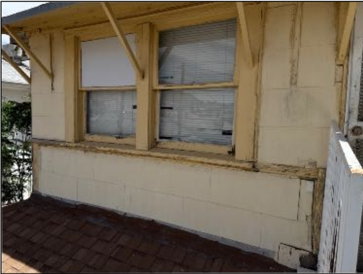
View of weathered wood on backside of structure walls
