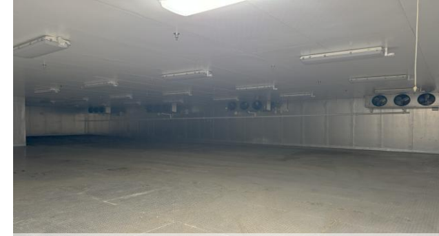
Cold Storage Area
