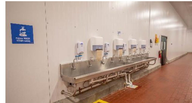
Hand washing station
