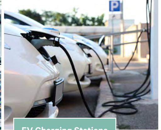
EV Charging Stations
