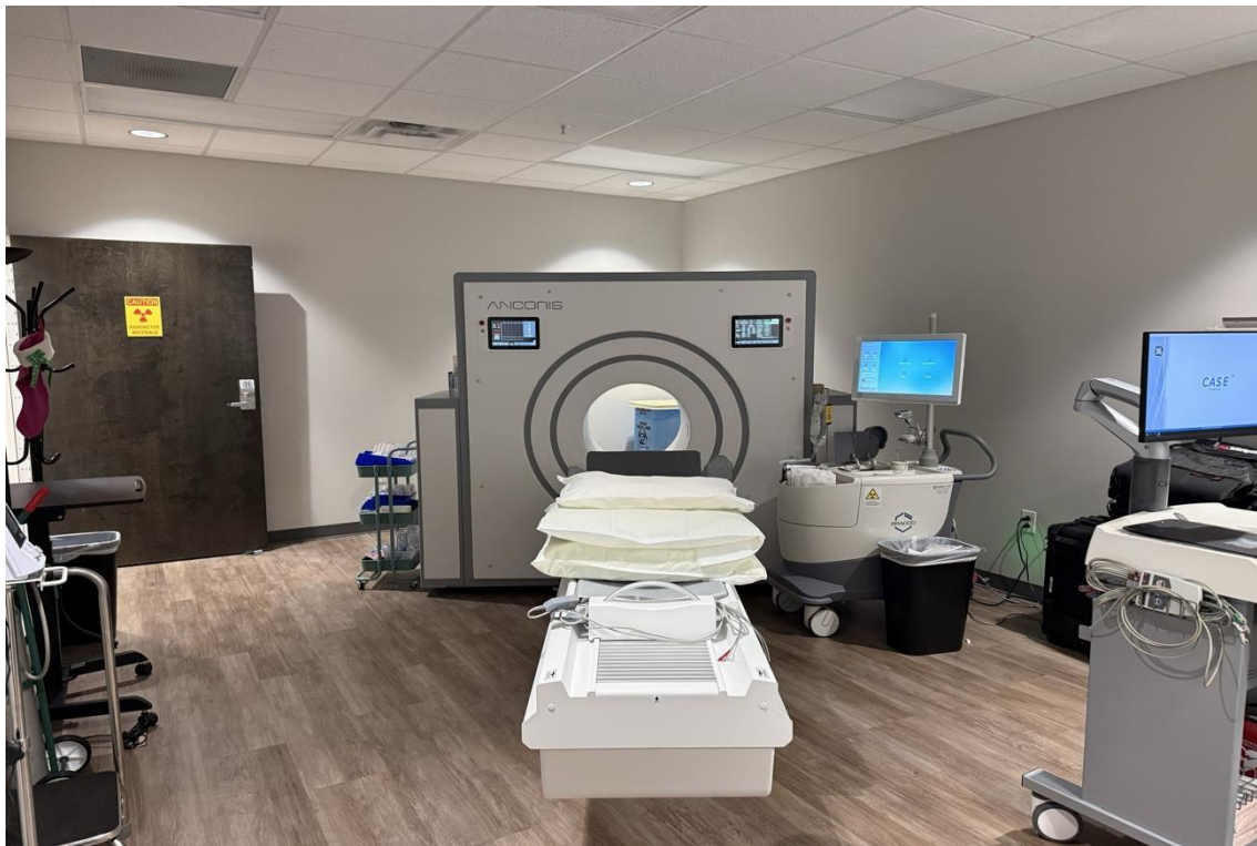
Nuclear medicine / PET-CT room with adjoining hot lab and shielded access
