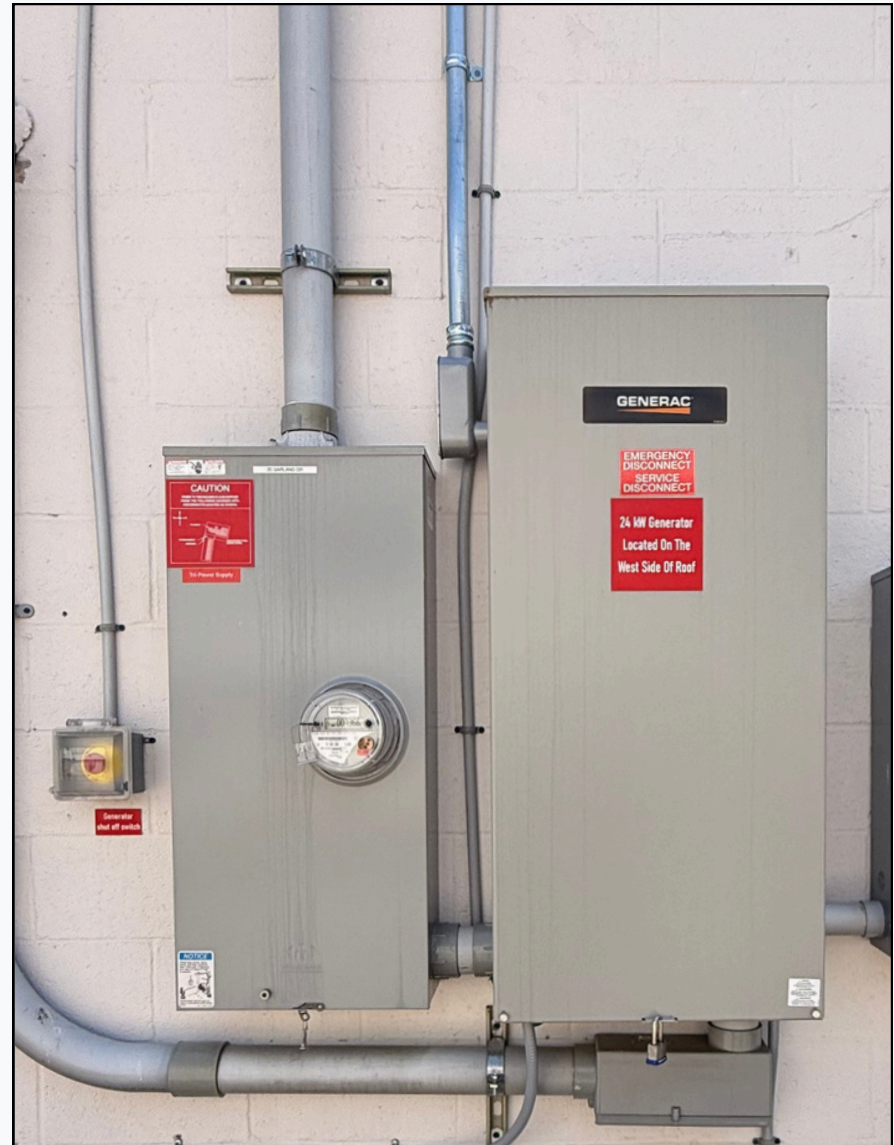
24KW Generator Provides Backup Power
