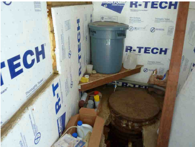
Interior small pump house
