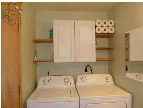
Laundry hoop ups in bathroom
