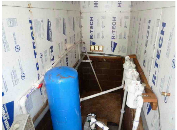
Interior larger pump house
