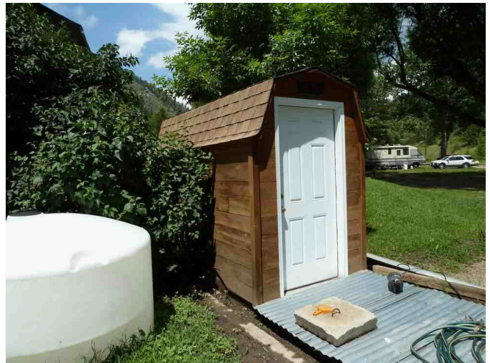
One of two Pump Houses
