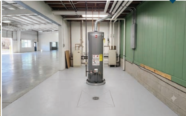
Hot Water Boiler
