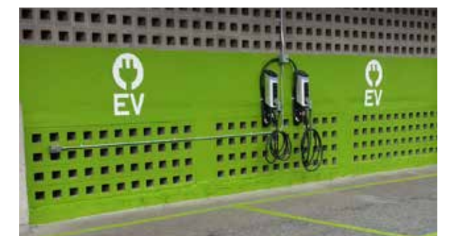
Two (2) electric vehicle charging stations
