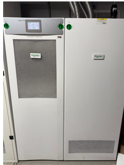
Battery Back Up 1 of 2
