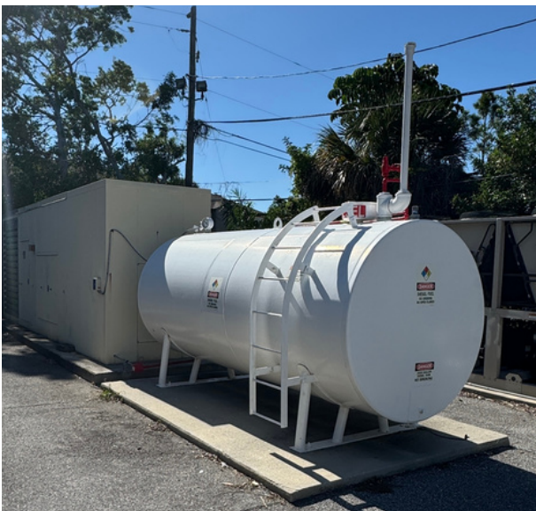
Ring Power Cat Generator w 2000 Gallon Diesel Tank
