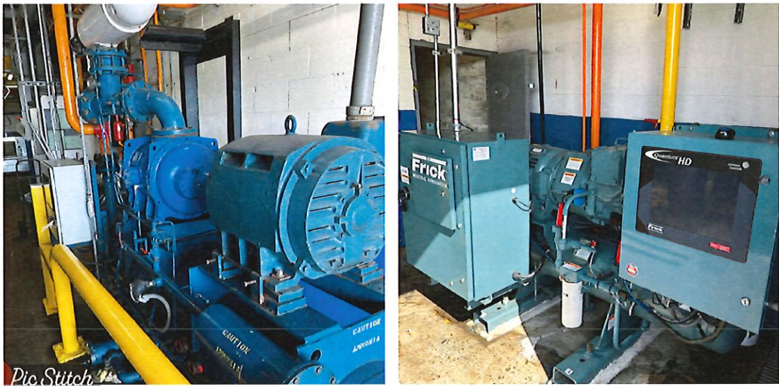
Refrigeration is in place for the freezing operations. A 150 HP low temp Howden screw compressor and a "brand new" Frick 70 HP is in place. For crab chilling and freezing, there are several chillers connected controlling temperatures of circulating water.
