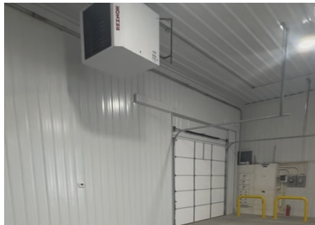
New Reznor heater & drive-in
