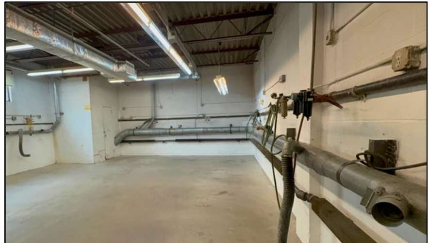
DUST COLLECTION SYSTEM
