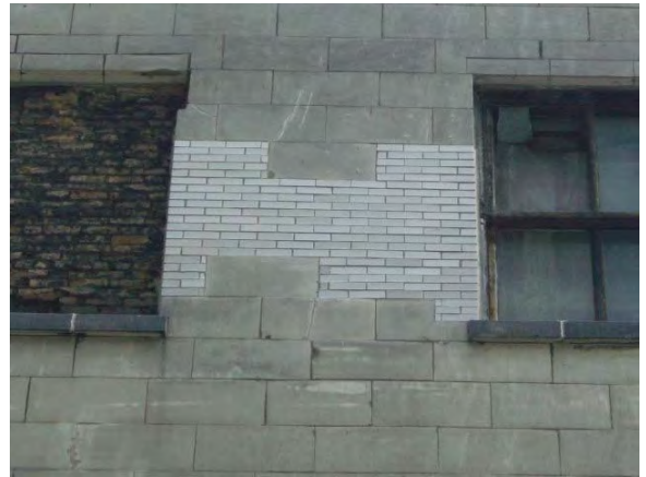
Image 124: Poor substitute cladding material and insensitive replacement of window.
