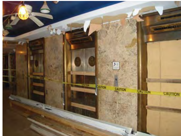
Image 62: Elevator lobby, first floor. Typical of all elevator doors on this floor.
