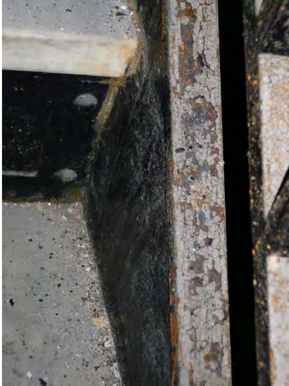
Image 71: Typical stringer condition, main stair, floors 2 and above.
