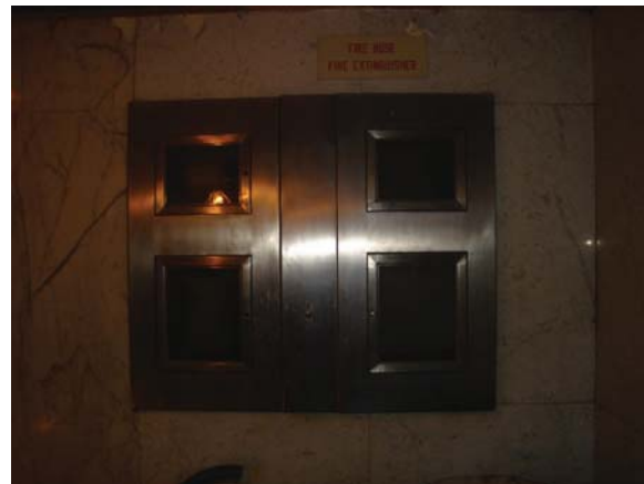
Image 54: Fire hose cabinet, main stairway, likely from 1951 remodeling.
