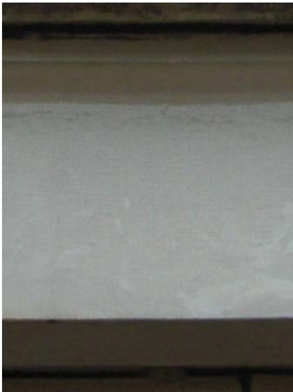
Image 125: Crazing evident in glazed finish of masonry units throughout the facades.
