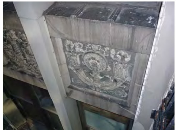
Image 26: Terra cotta detail, north façade between 3 rd and 4 th floors.
