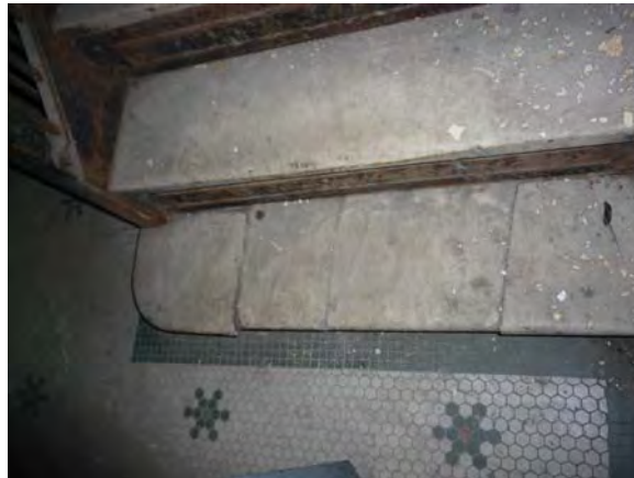
Image 114: West stair, typical condition from first basement to first floor.
