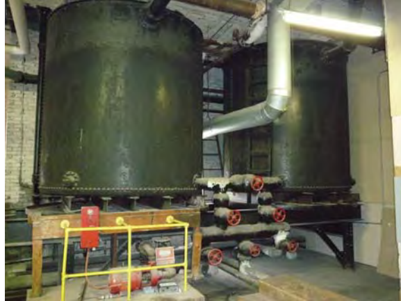
Image 96: Mechanical equipment, 22 nd floor.
