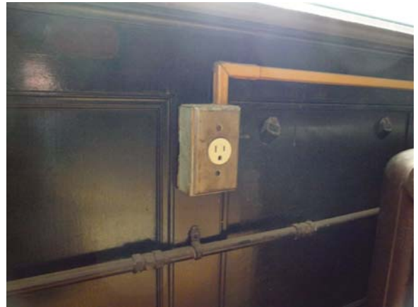
Image 110: Typical electric conduit/outlet, 20 th floor, southeast suite.
