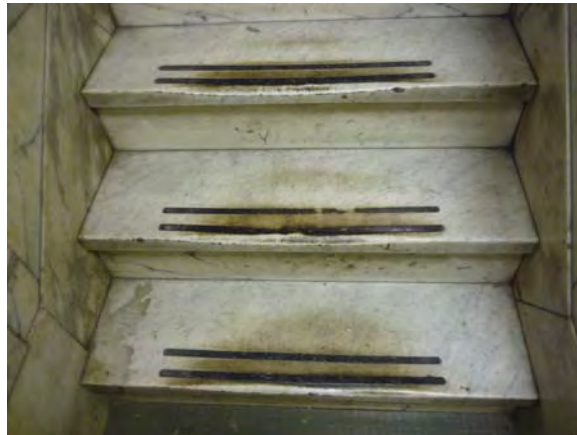
Image 106: Wear on marble stairs between first floor and first basement.
