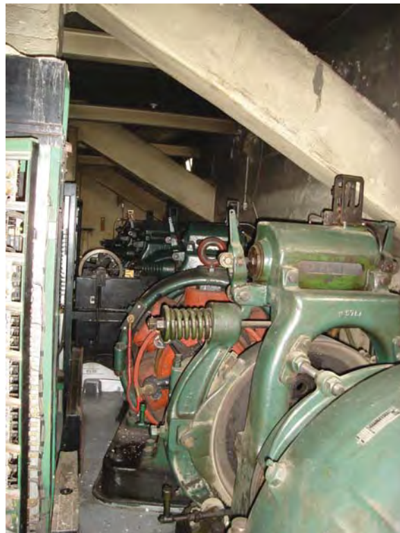
Image 98: Elevator equipment, 22 nd floor.
