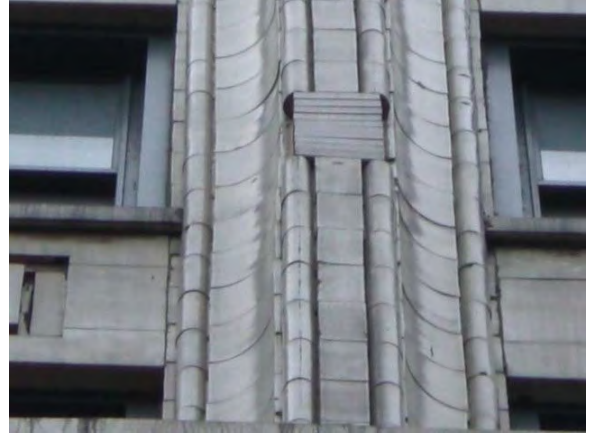
Image 116: Poor substitution of glazed brick for terra cotta, east façade.
