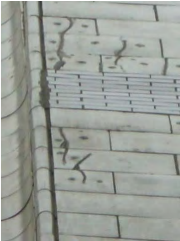
Image 117: Poor substitute cladding material and failure of surrounding terra cotta.
