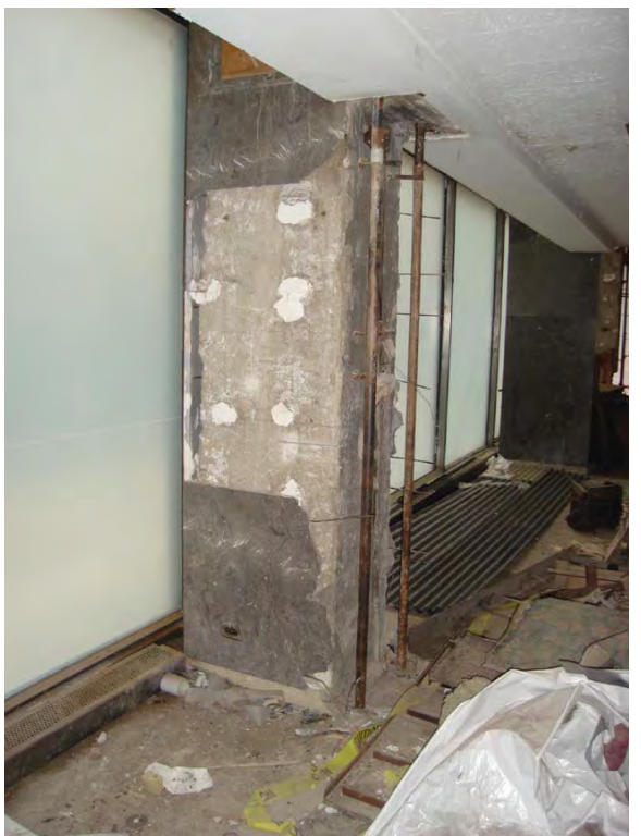
Image 66: Typical condition of columns along the north and east facades on the first floor.
