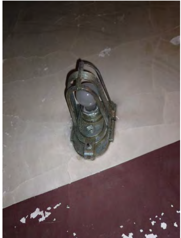
Image 48: Wall sconce, 16 th floor stair.
