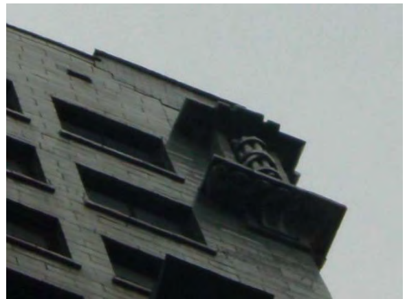
Image 126: Failing parapet corner with cracking evident in terra cotta.
