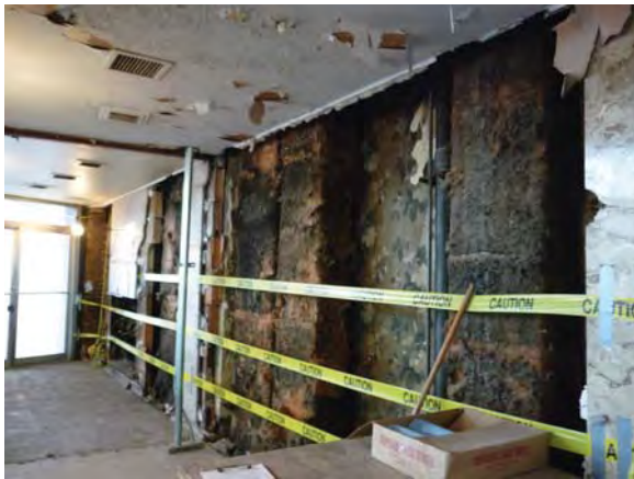
Image 63: South wall of main lobby. Much of the 1951 marble cladding has been removed.
