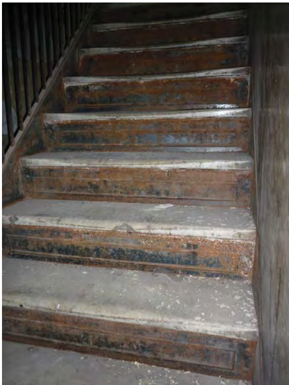
Image 113: West stair, typical condition from first basement to first floor.
