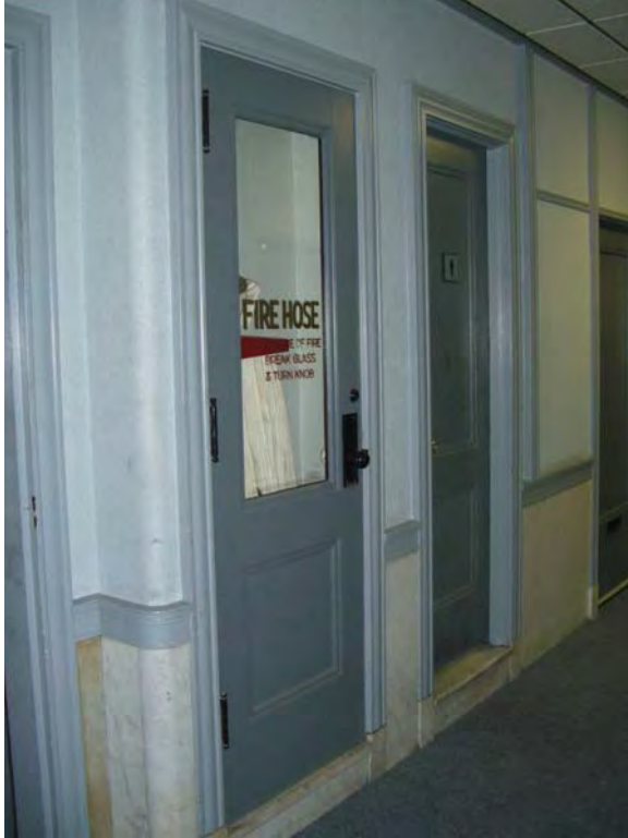
Image 83: Fire hose closet, typical of floors 2 through 21.
