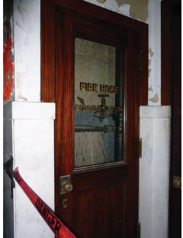
Image 56: Fire hose closet door, 15 th floor. Typical of floors 2 through 15.
