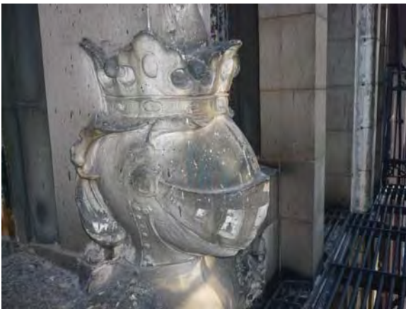
Image 25: Terra cotta detail, north façade between 3 rd and 4 th floors.
