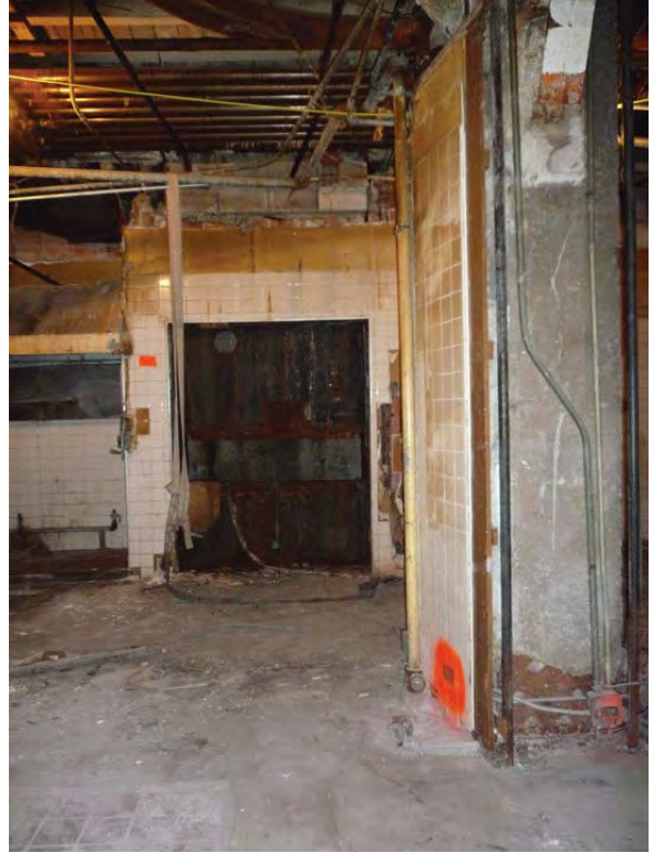
Image 40: First basement, freight elevator.
