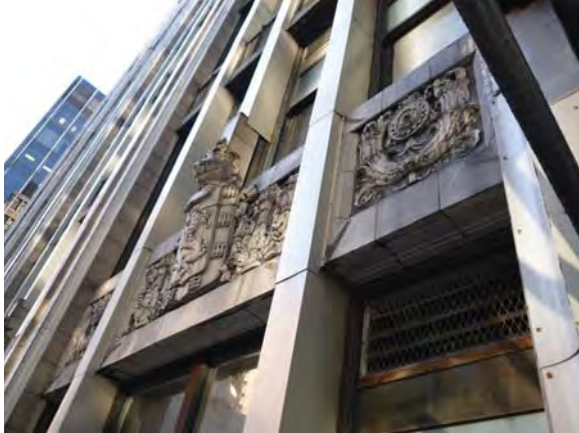
Image 19: Terra cotta detail, north façade between 3 rd and 4 th floors.
