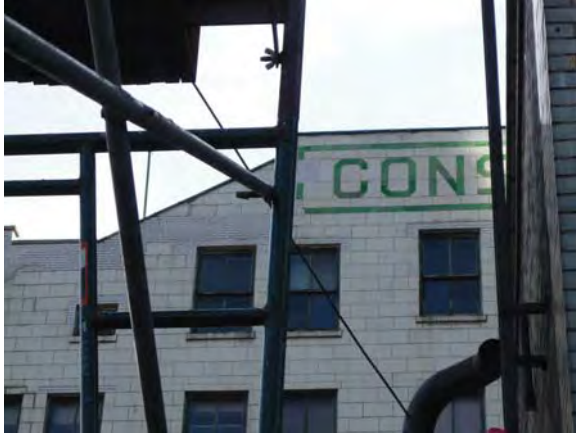
Image 107: Typical façade conditions showing varied types of patching repairs.
