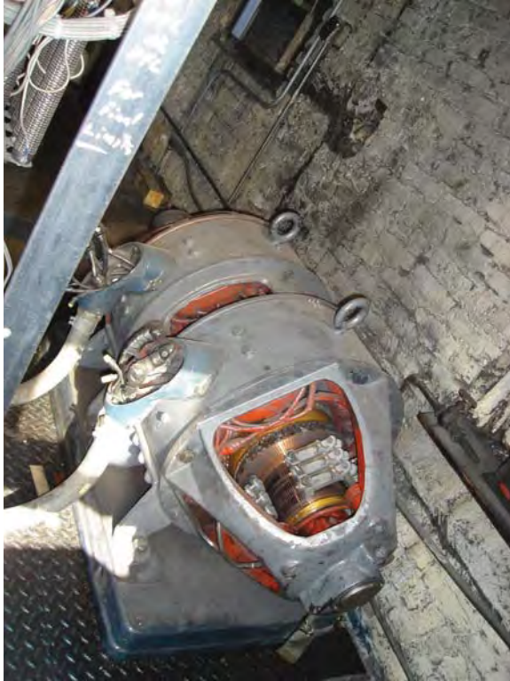
Image 95: Elevator equipment, freight elevator penthouse.
