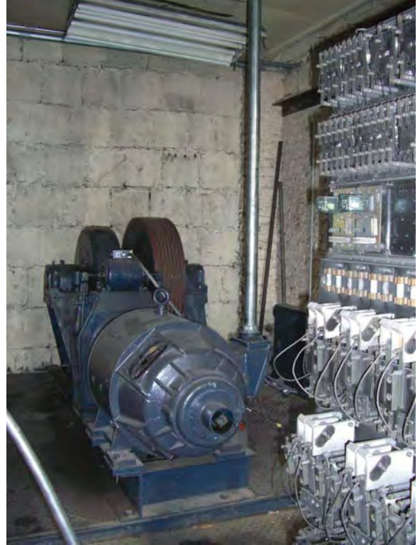
Image 100: Elevator equipment, freight elevator penthouse.
