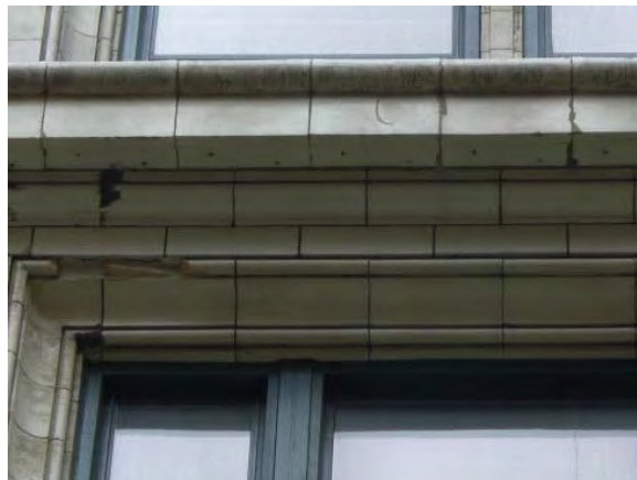
Image 122: Delamination of terra cotta due to stresses in the failing lintel.
