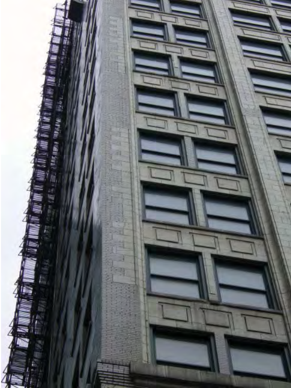
Image 115: Poor substitution of glazed brick for terra cotta, southwest corner.
