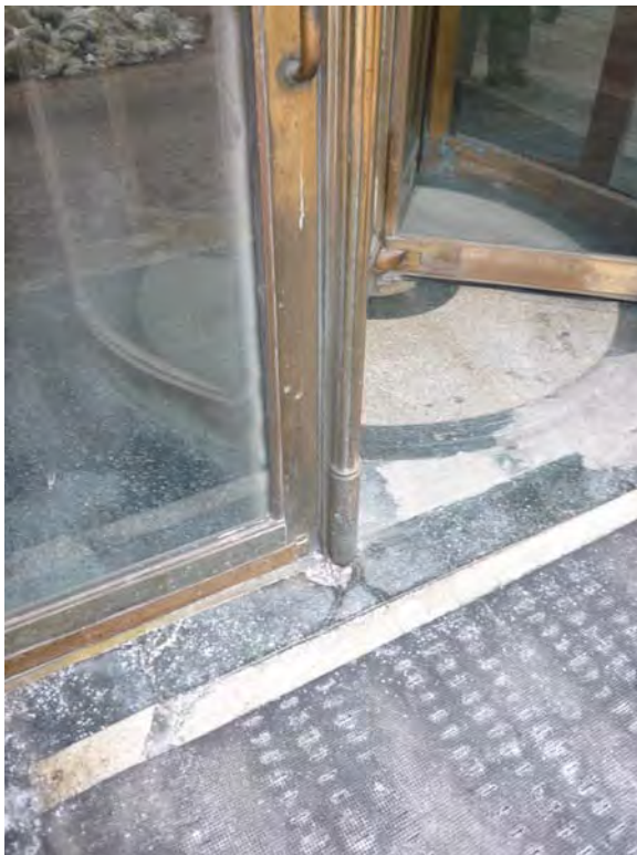
Image 109: Worn terrazzo, main entry.
