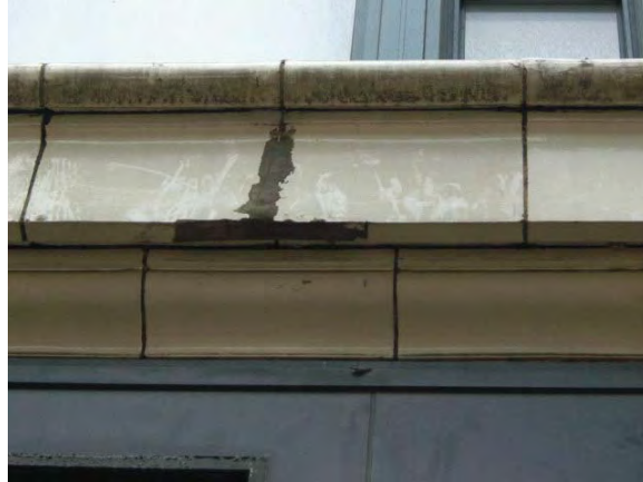
Image 120: Improper repair of failing terra cotta.
