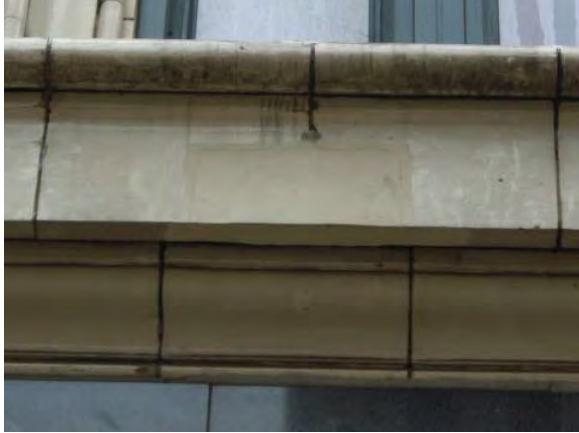
Image 119: Unsightly mortar patch. Doomed to fail.
