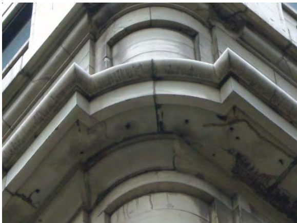
Image 121: Stresses in terra cotta due to anchor failure and stresses in wall. Poor substitution of glazed brick for terra cotta and improper patching also evident.
