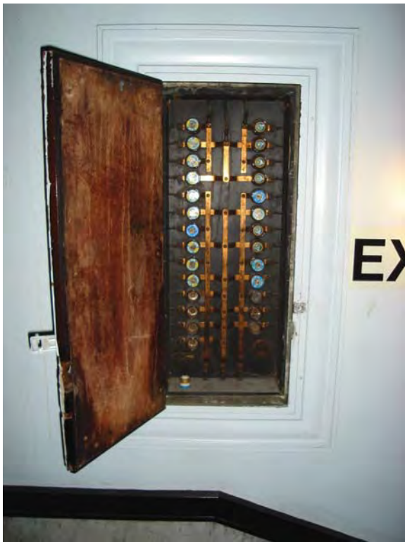
Image 97: Circuit box, 9 th floor.
