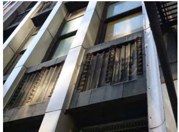
Image 24: Typical terra cotta detail of the 4 th through 15 th floors, north façade.
