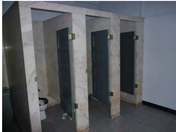
Image 90: Typical restroom stall partitions.
