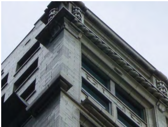
Image 123: Delamination of terra cotta unit due to stresses in the failing lintel.
