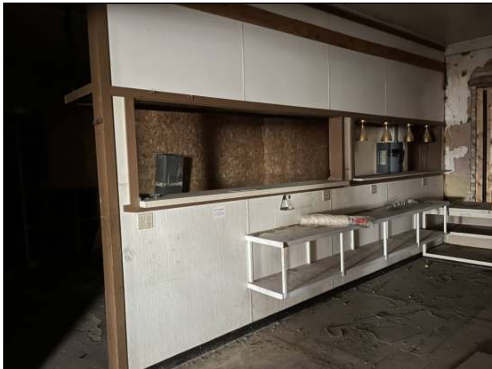
8 : Alternative view of the deli area on the first floor of the Subject Property.
