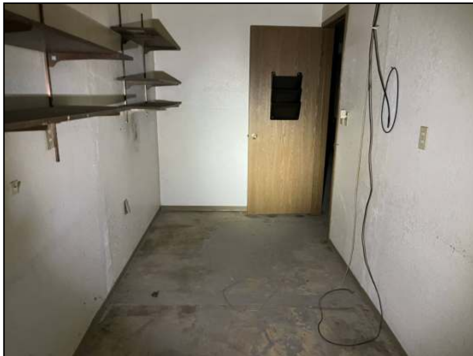
12 : View of the storage room on the first floor of the Subject Property.
