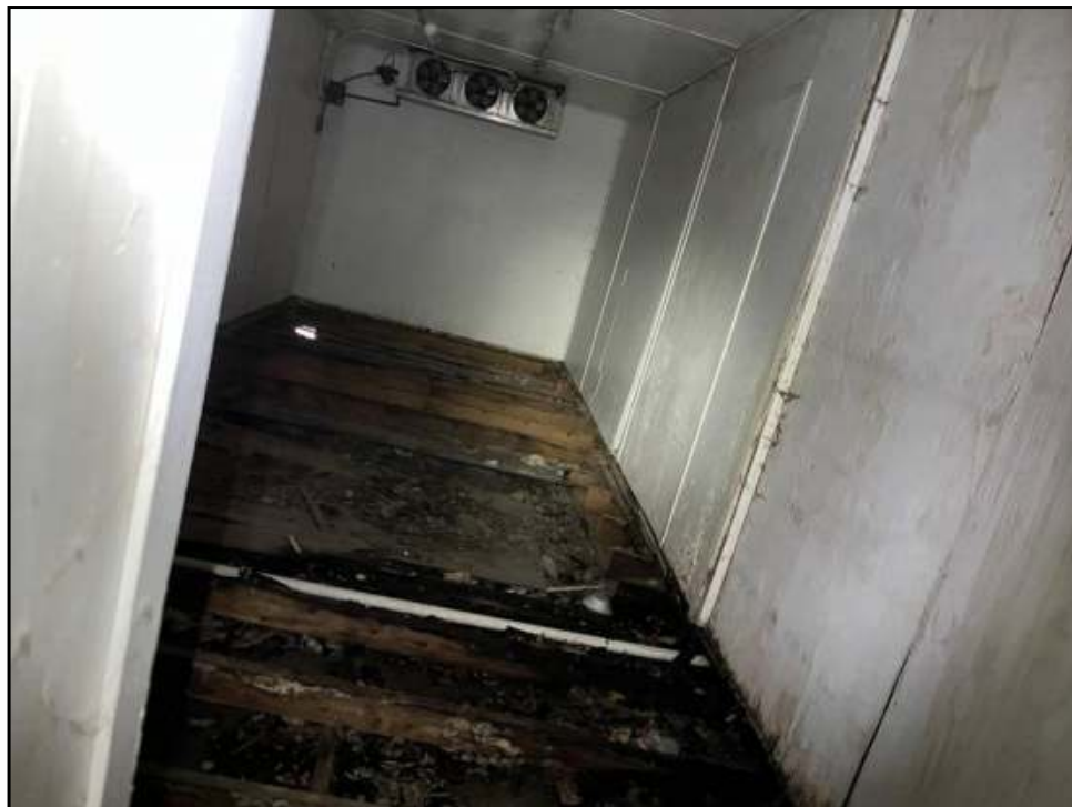
14 : View of the walk-in cooler on the first floor of the Subject Property.
