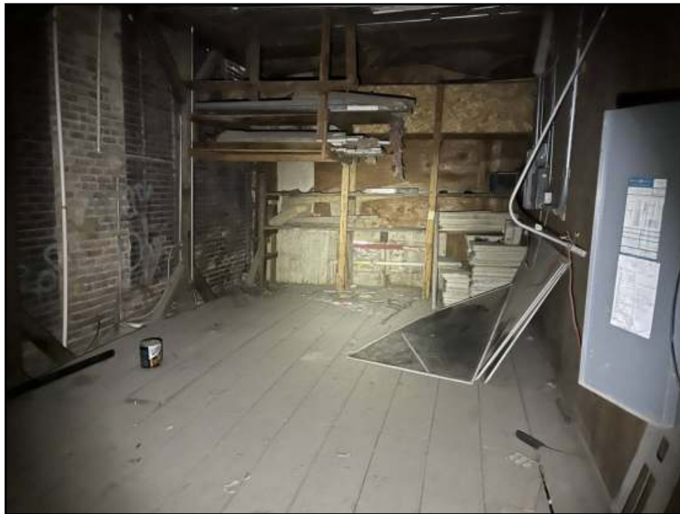
15 : View of the back room storage area on the first floor of the Subject Property.
