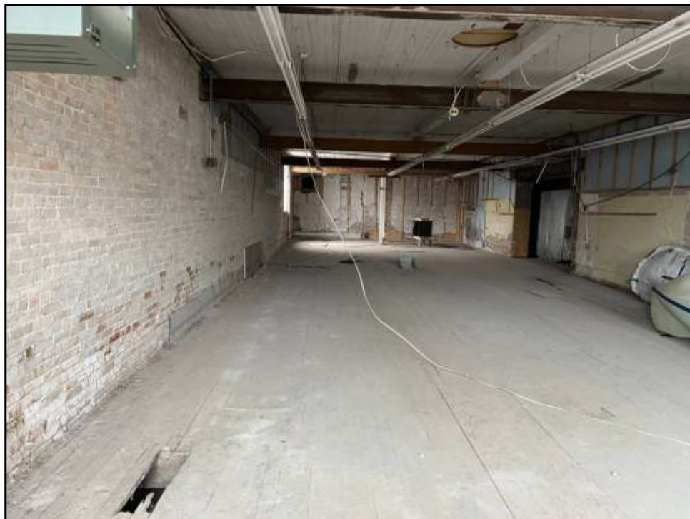
2 : View of the primary restaurant area on the first floor of the Subject Property.
