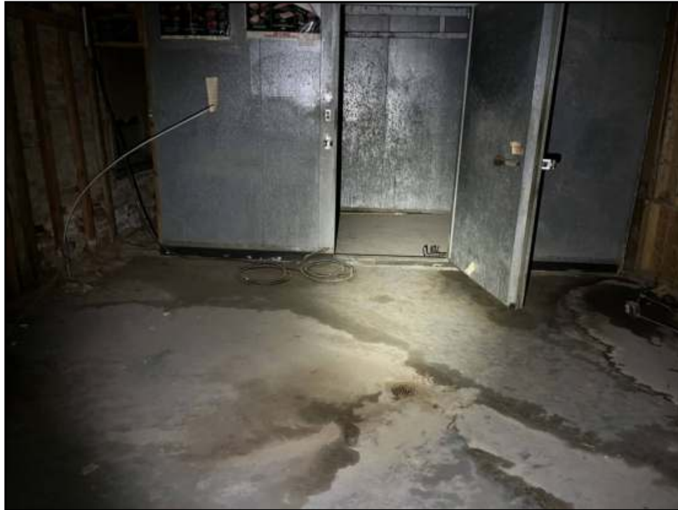
9 : View of the walk-in freezer on the first floor of the Subject Property.
