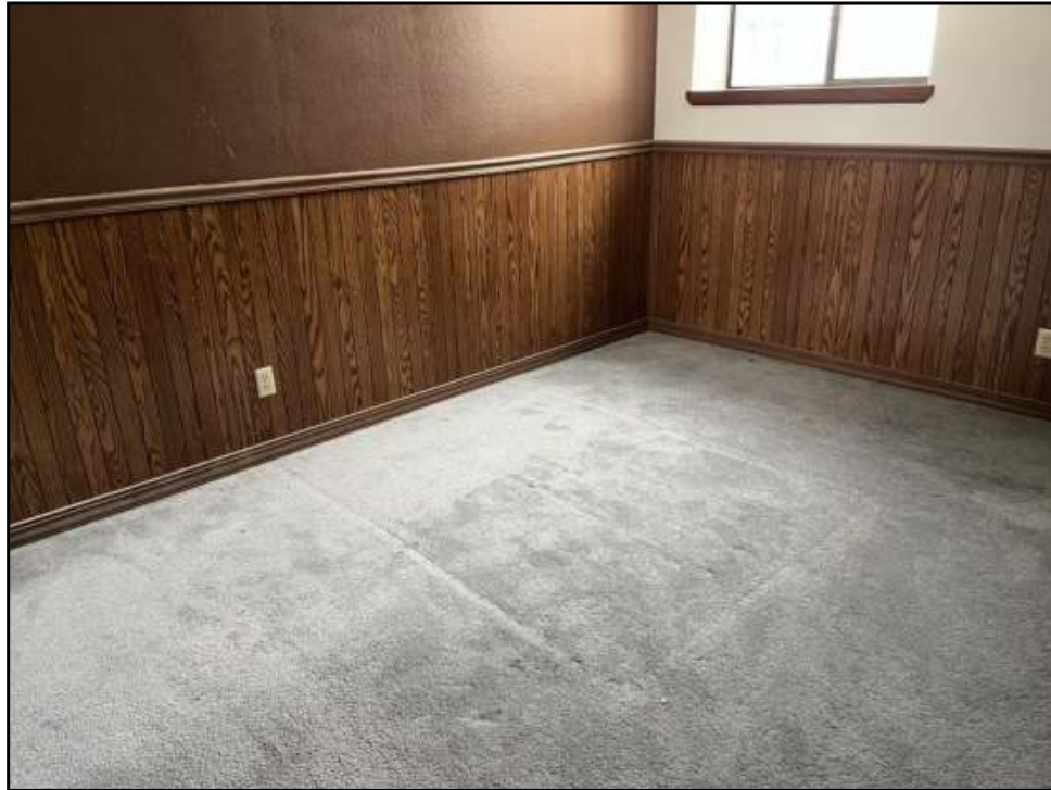
21 : View of the bedroom on the second floor of the Subject Property.
