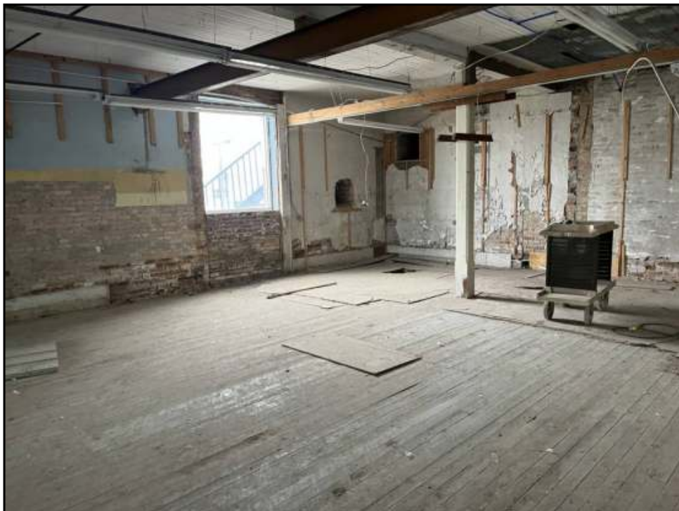
4 : Alternative view of the primary restaurant area on the first floor of the Subject Property.
