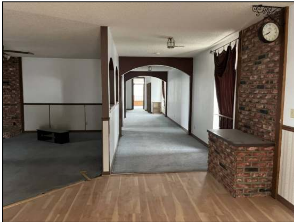
19 : View of the hallway on the second floor of the Subject Property.
