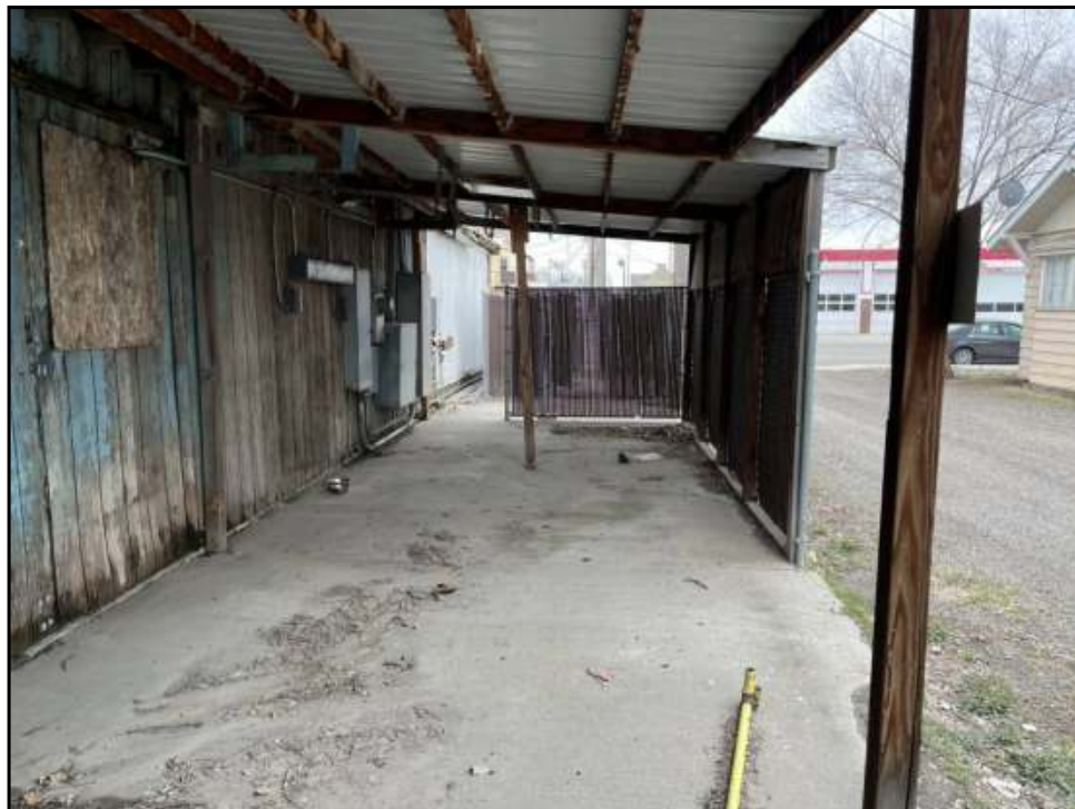
16 : View of the southwest side of the structure on the Subject Property.
