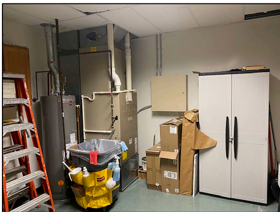
Mechanical closet (new hot water heater with floor drain).
