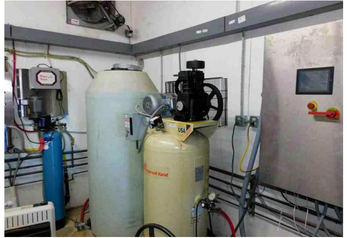
WATER TREATMENT & COMPRESSORS
