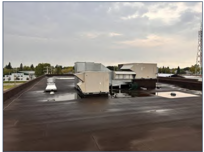
View of rooftop HVAC systems.
