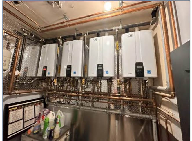
Main Level: Mechanical room.
