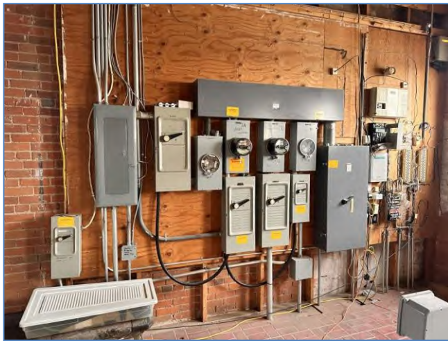
Second Level: 800-Amp power panel with sub-panels.
