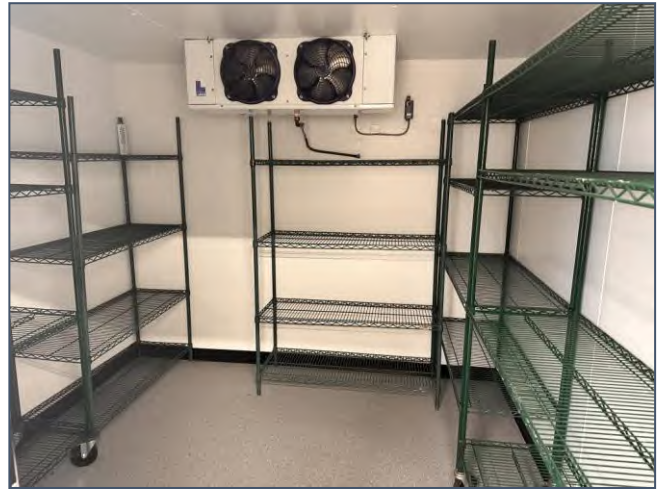
Main Level: Built-in walk-in cooler.
