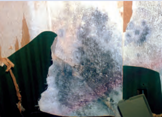
Photo 5: Mold growth behind wallpaper
