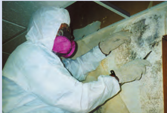
Photo 7: Remediation worker with limited PPE
