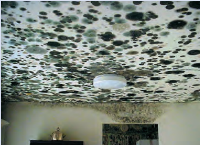
Photo 2: Extensive mold contamination of ceiling and walls
