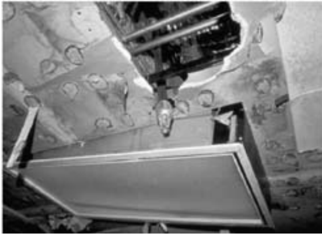
Figure 57 - A broken sprinkler pipe caused extensive water damage after it was sheared off by ceiling movement in the 1994 Northridge Earthquake.
