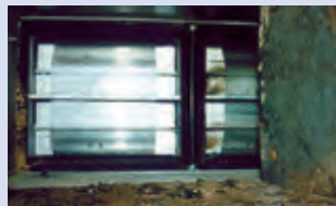
Photo 4C: Moldy air duct
