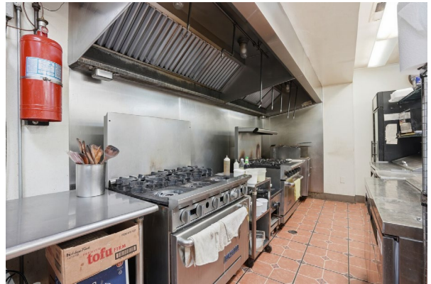
Cooking line with hood and suppression
