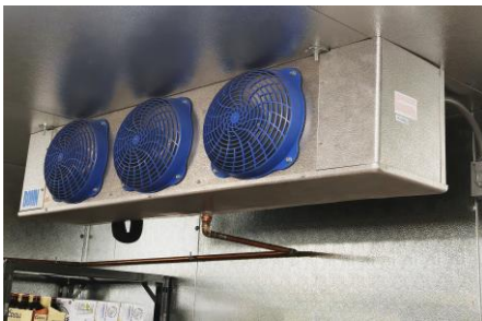
Walk-in cooler — insulated box with ceiling evaporator
