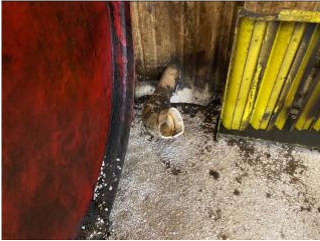
Two-inch PVC pipe located on the southern wall of the automotive garage connecting to an exterior waste oil AST.
