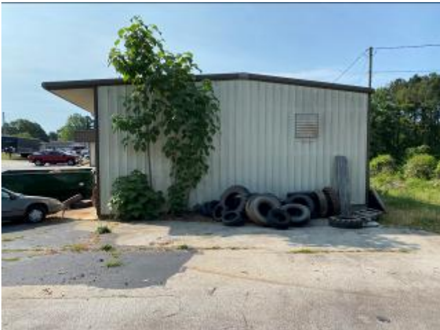
Used tires observed along the west side of the automotive garage.
