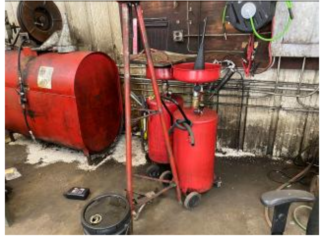
Twenty-gallon lift drains observed in the automotive garage.
