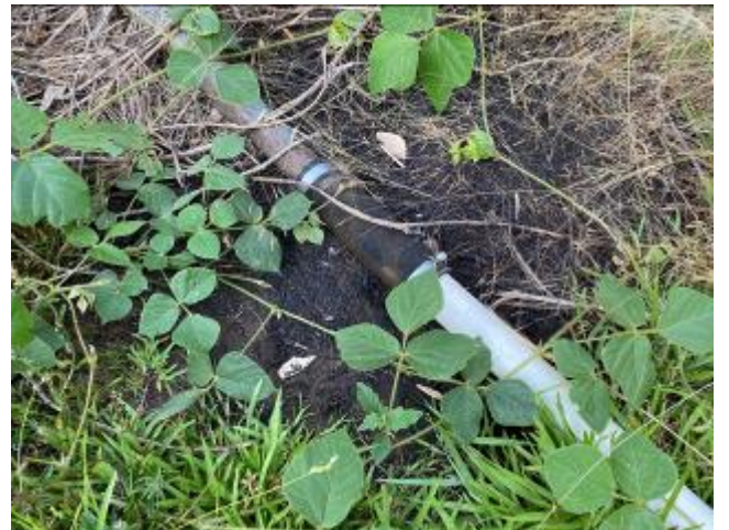
Oil-stained and stressed vegetation beneath the PVC drain pipe from the automotive garage to the exterior waste oil AST.
