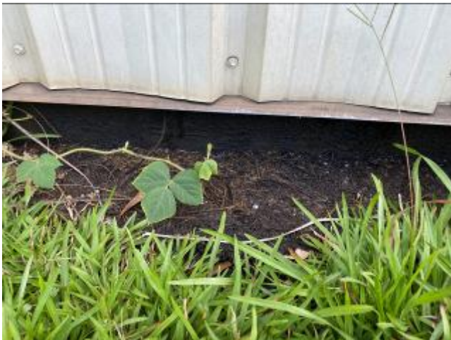
Oil-staining and stressed vegetation observed along the exterior foundation along the south side of the automotive garage.
