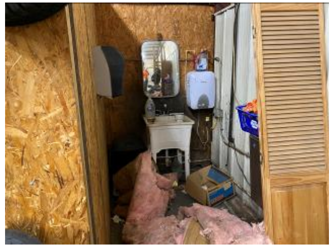
Shop sink located in the tire storage area in the building.
