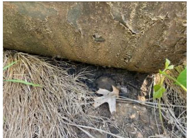
Oil-stained and stressed vegetation observed beneath the former waste oil AST.
