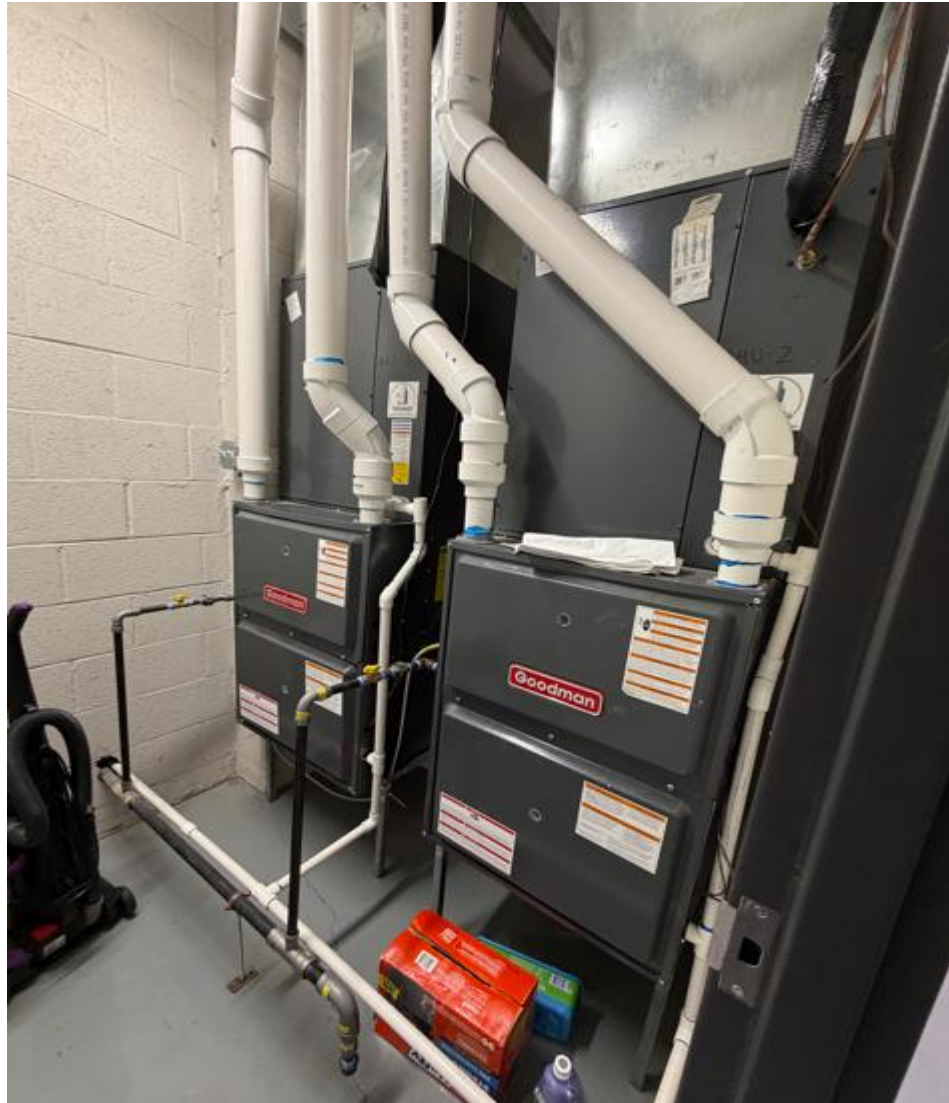
HVAC: 2- 5 ton Split Systems
