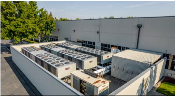
MECHANICAL EQUIPMENT YARD COOLING UNITS AND BACKUP GENERATOR
