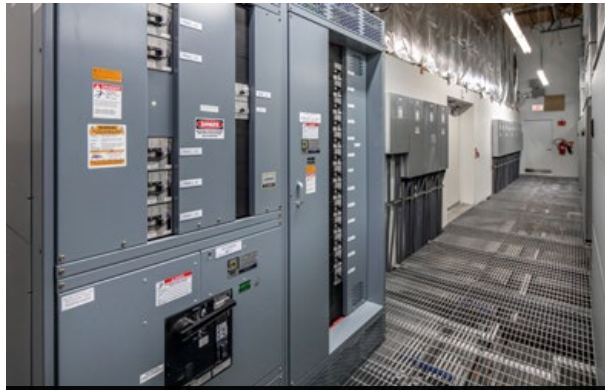
MECHANICAL CORRIDOR ELECTRICAL AND LAB FIRE SUPPRESSION
