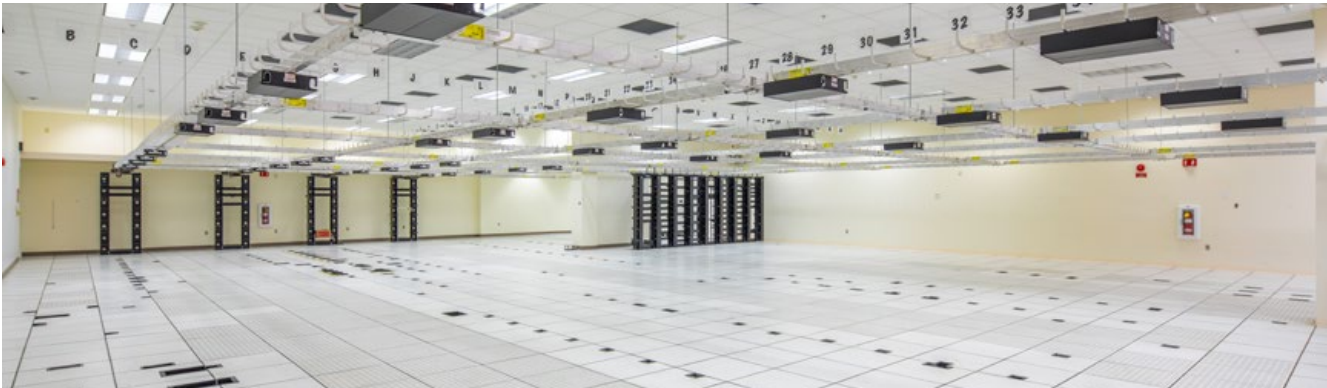
DATA CENTER / LAB AREA WITH 2-FOOT RAISED FLOORS
