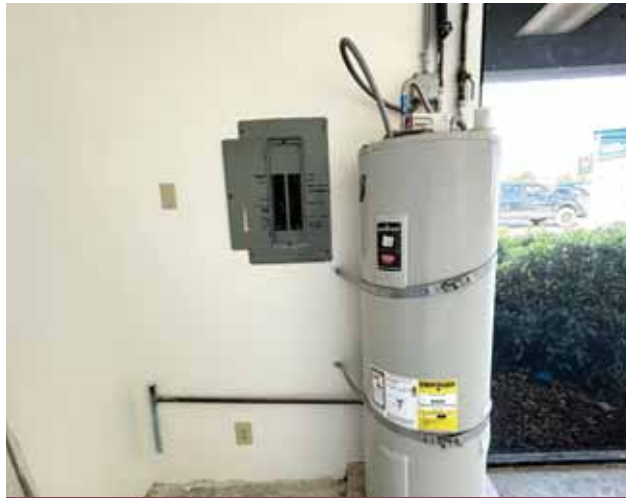
Electrical Panel & 40-Gallon Electric Hot Water Heater
