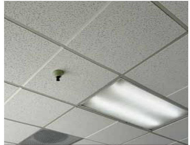
3093 McKee Road - Fire Sprinklered
