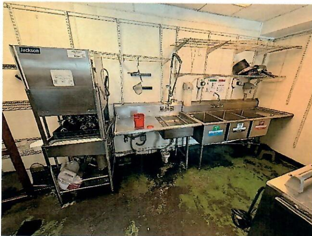
Dishwasher and 3 compartment sink
