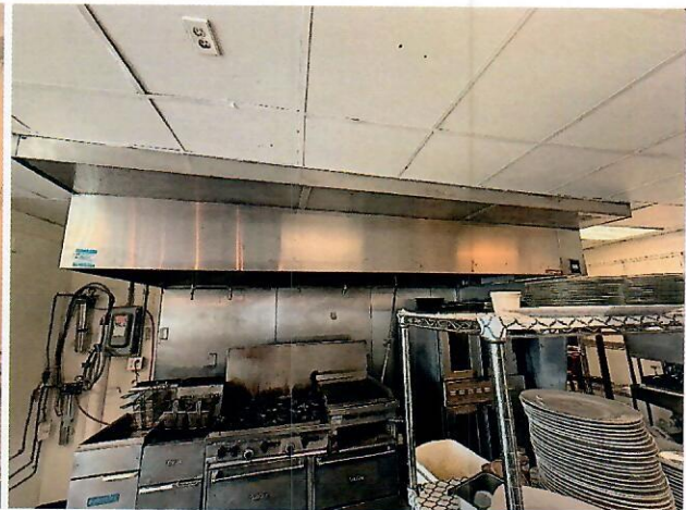
12 foot hood system and equipment
