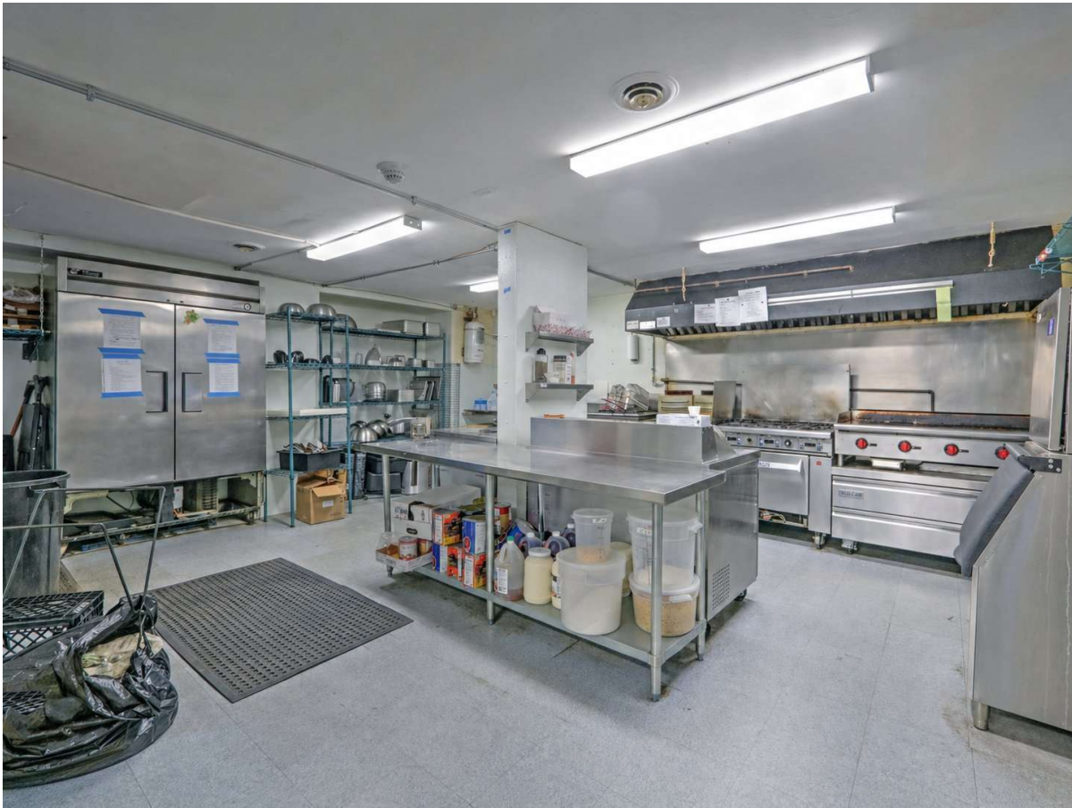
Full commercial kitchen — hood, 6-burner range, flat-top, walk-in cold storage
