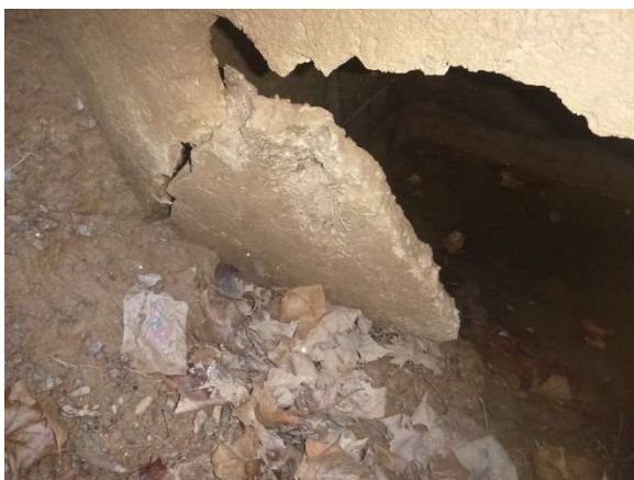
Failed wall of existing Cistern adjacent to sinkhole
