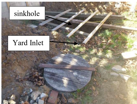
View of secured area of failed Cistern and resulting sinkhole
