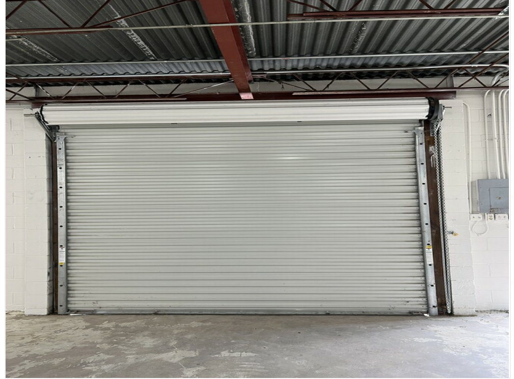
Unit B - Insulated Roll Up Door
