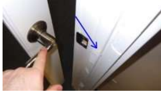
Door stop doesn't stop door.
