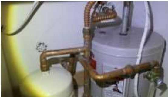
9220 water heater in bathroom.
