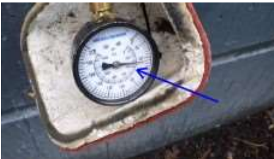
45 PSI at exterior hose bib.
