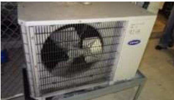
9218 heat pump in garage below.
