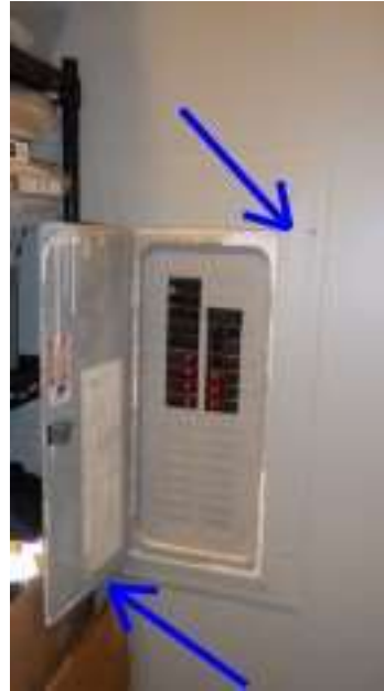
Missing dead-front panel screws.
