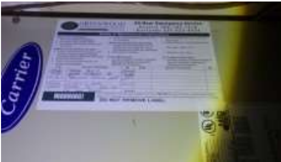
9220 air handler above the ceiling tiles.
