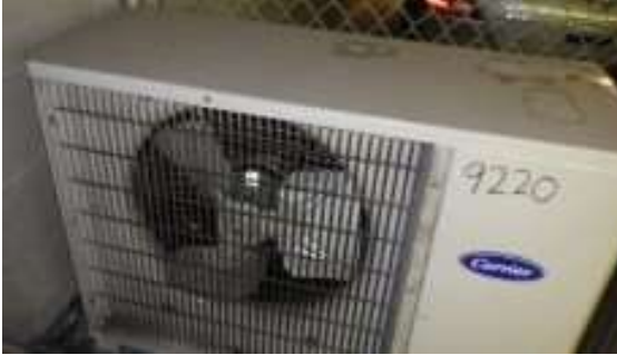
9220 heat pump in garage below.
