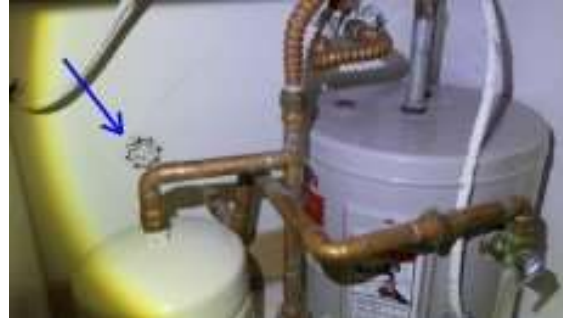
Water shut off beneath bathroom sink in 9220.
