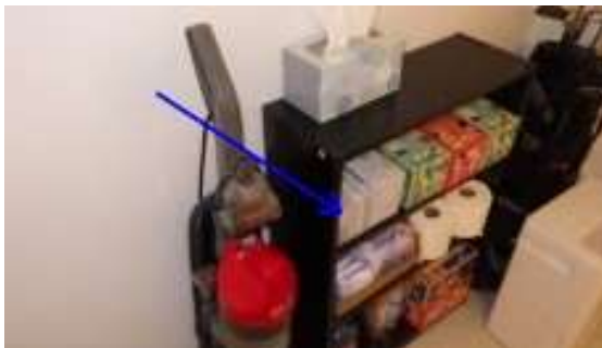
Outlet behind cabinet in 9218 bathroom is not GFCI protected.
