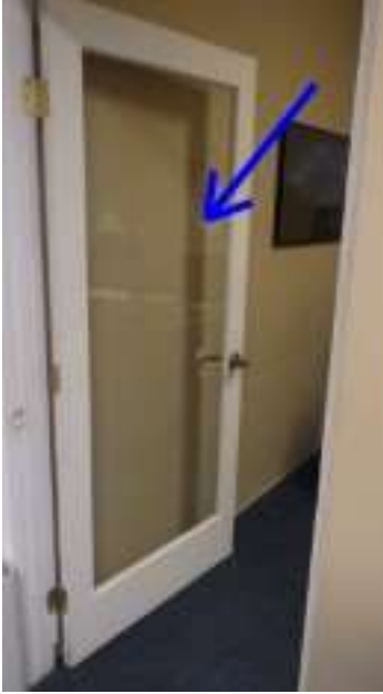
Office door is difficult to latch.
