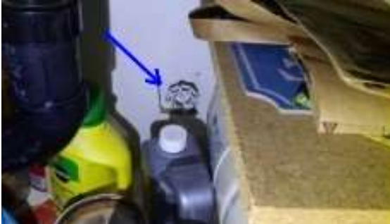
Water shut off beneath sink in 9218.
