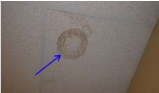
Discoloration noted in ceiling tile above the entrance.
