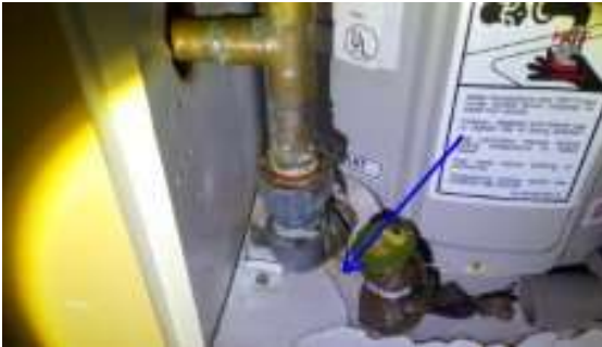
Oxidation and previous moisture noted.
