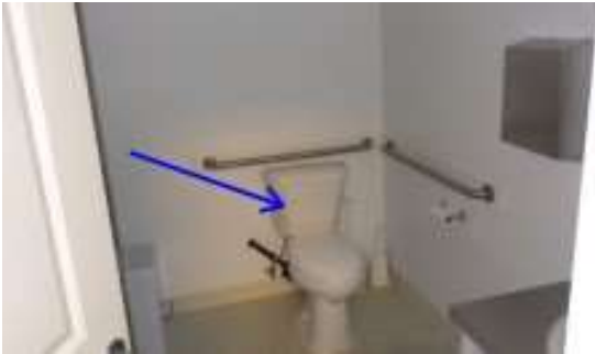
Toilet runs after being flushed.
