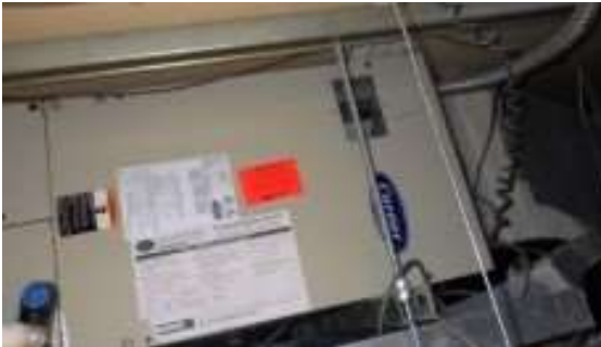
9218 air handler above the ceiling tiles.
