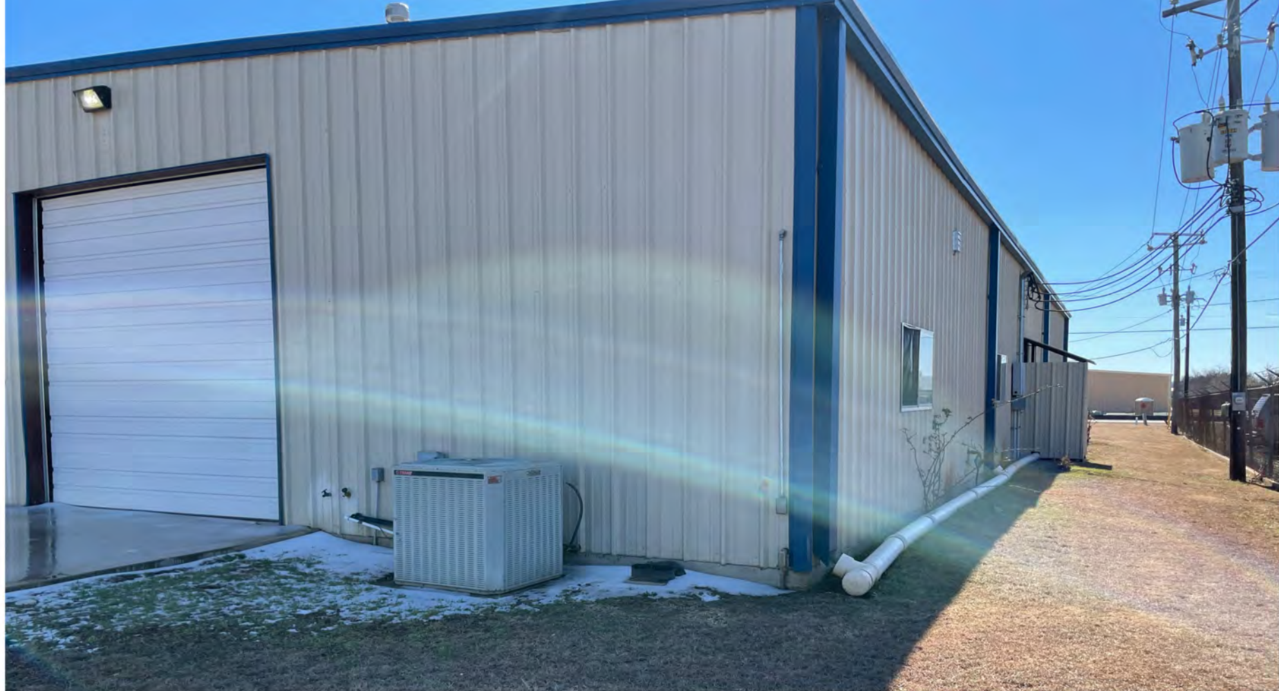
NORTHWEST CORNER OF BLDG (LOOKING OUT TO FM 2093 WITH EVIDENCE OF RARE TEXAS SNOW
