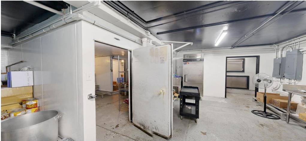
Basement walk-in cooler and cold storage
