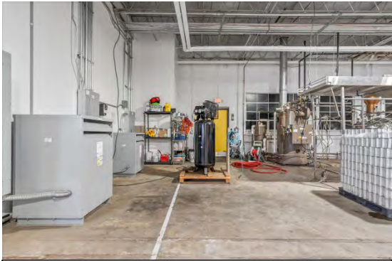
View of Inside Power
