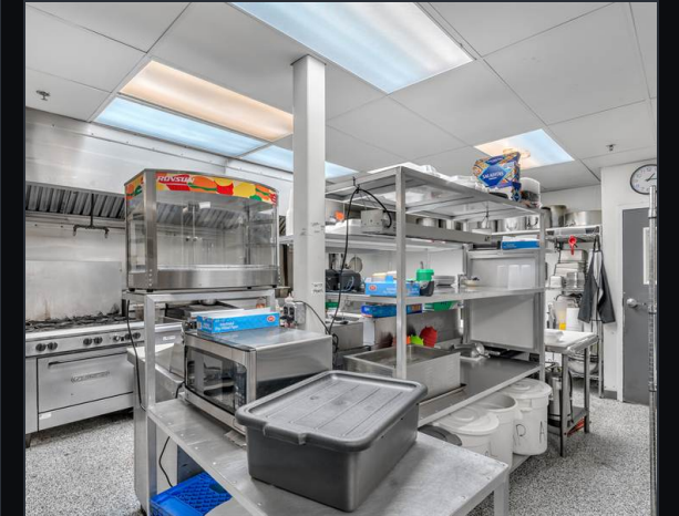
COMMERCIAL KITCHEN Full build-out, hooded cook line
