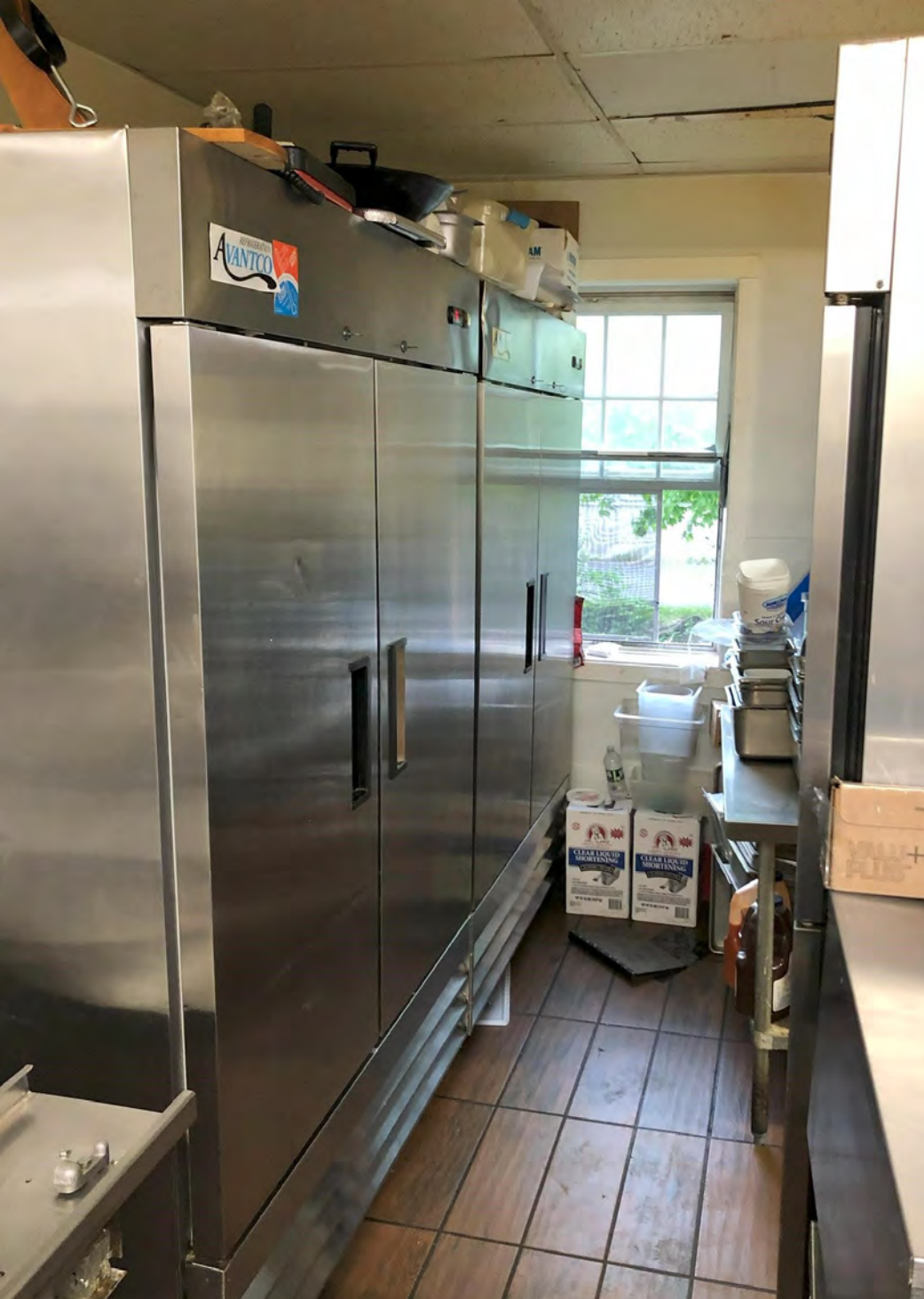
Kitchen - commercial refrigerator
