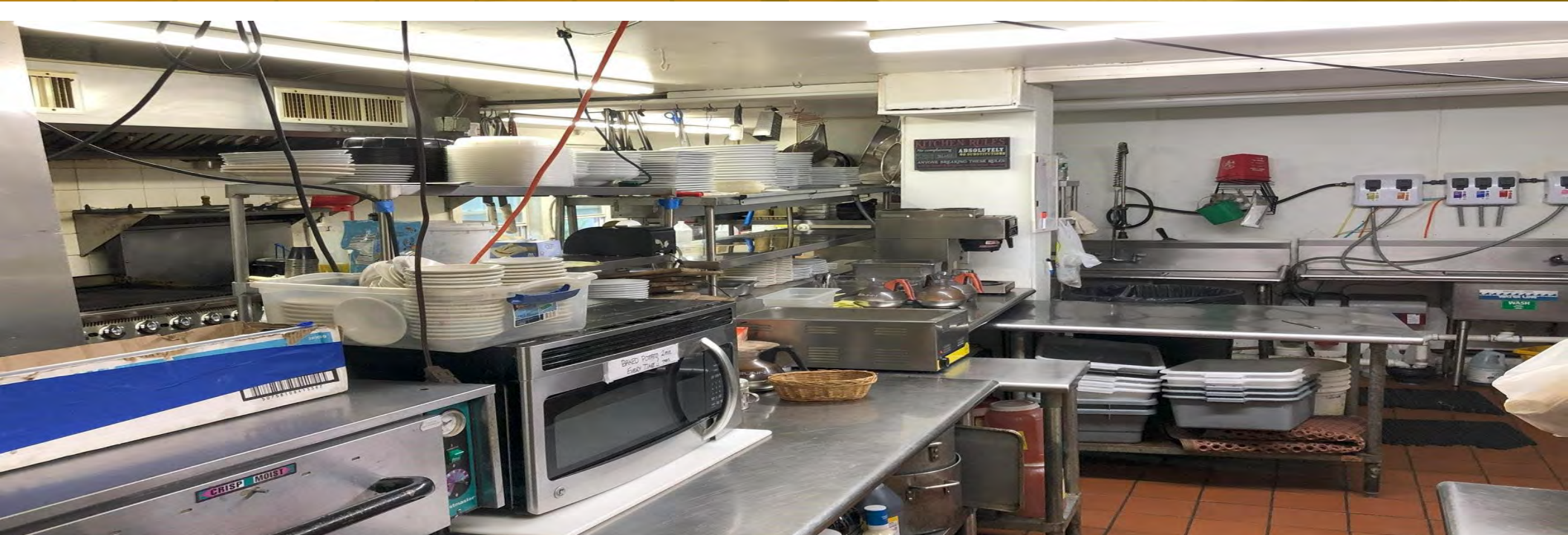
Kitchen - countertop equipment & sink
