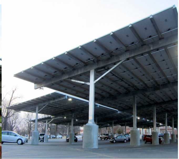
Solar Panel Covered Parking
