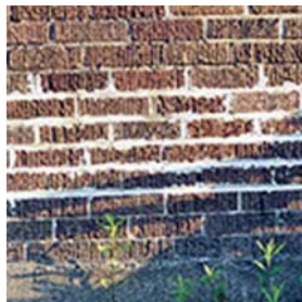
Inappropriate mortar work
