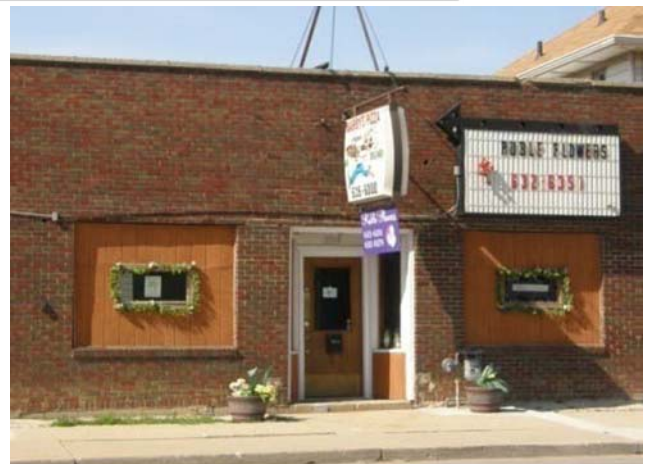
Filling in windows detracts from the architectural integrity of the building.
