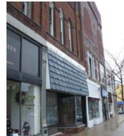
Inappropriate materials and use of Mansard roofing.
