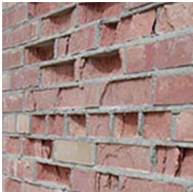
Excessively deteriorated brick
