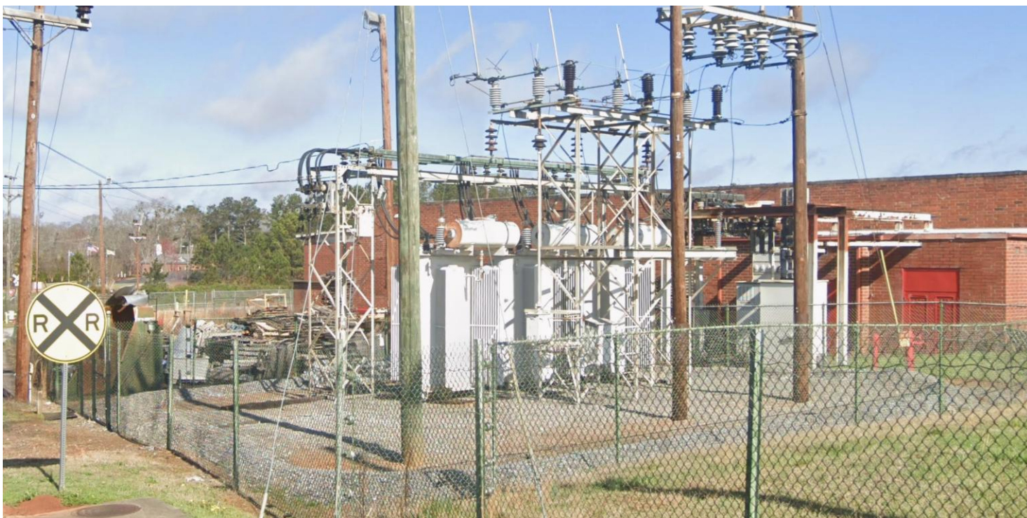
Existing Duke Energy Utility Substation / Transformer Yard Located On-Site
