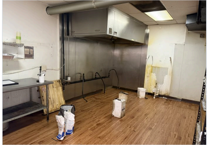
Commercial exhaust hood with gas drops for cooking equipment
