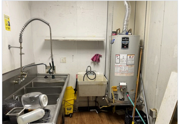
Three compartment sink with pre rinse, mop sink, and water heater
