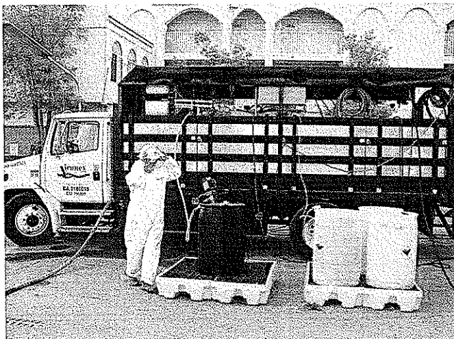
Sulfuric Acid and Hydrogen Peroxide separated in secondary containment, staged for injection
