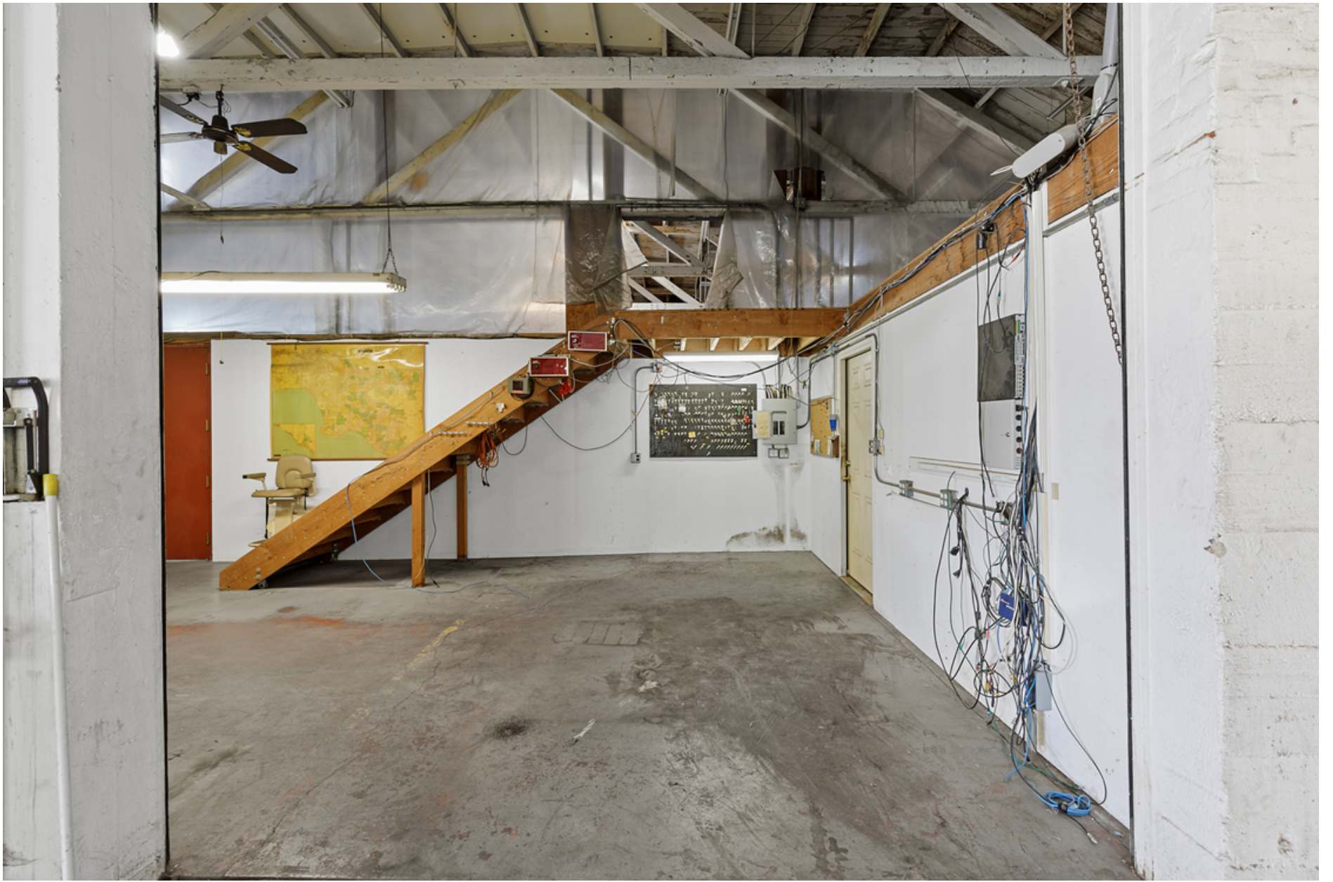
Workshop Area - Utility Access
