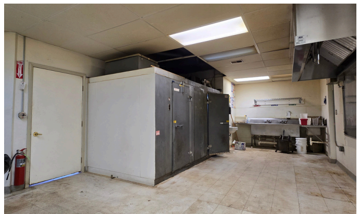
Commercial Kitchen & Walk-In Cooler
