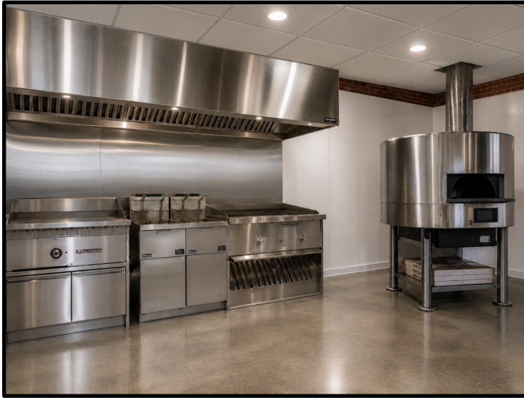
Kitchen; Newly Installed Range Hood & Rotary (multi-use) Pizza Oven
