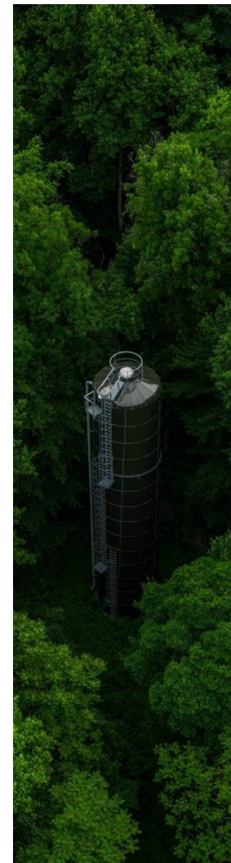
Water storage tank, installed.
